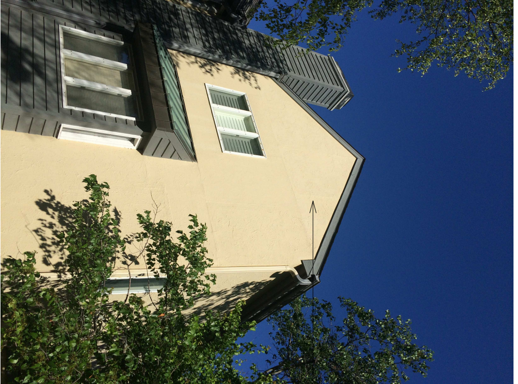
Exterior Facade - showing typical "telegraphing" of sheathing through EIFS finish
