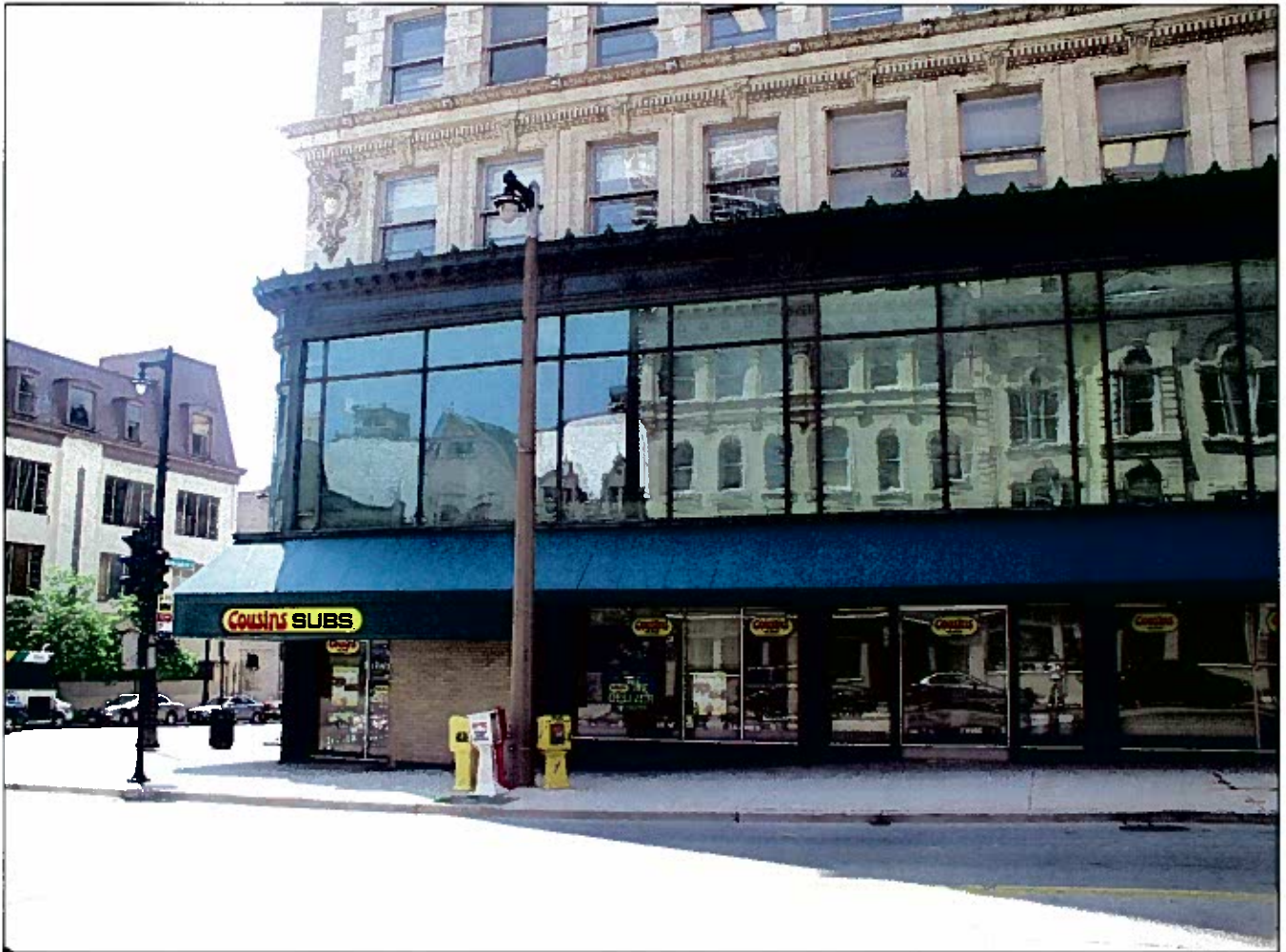
324 E. Wisconsin Ave. 071660 7-7-08 Looking Westerly on North Milwaukee Street at the lower Brick wall on the south side of the building
