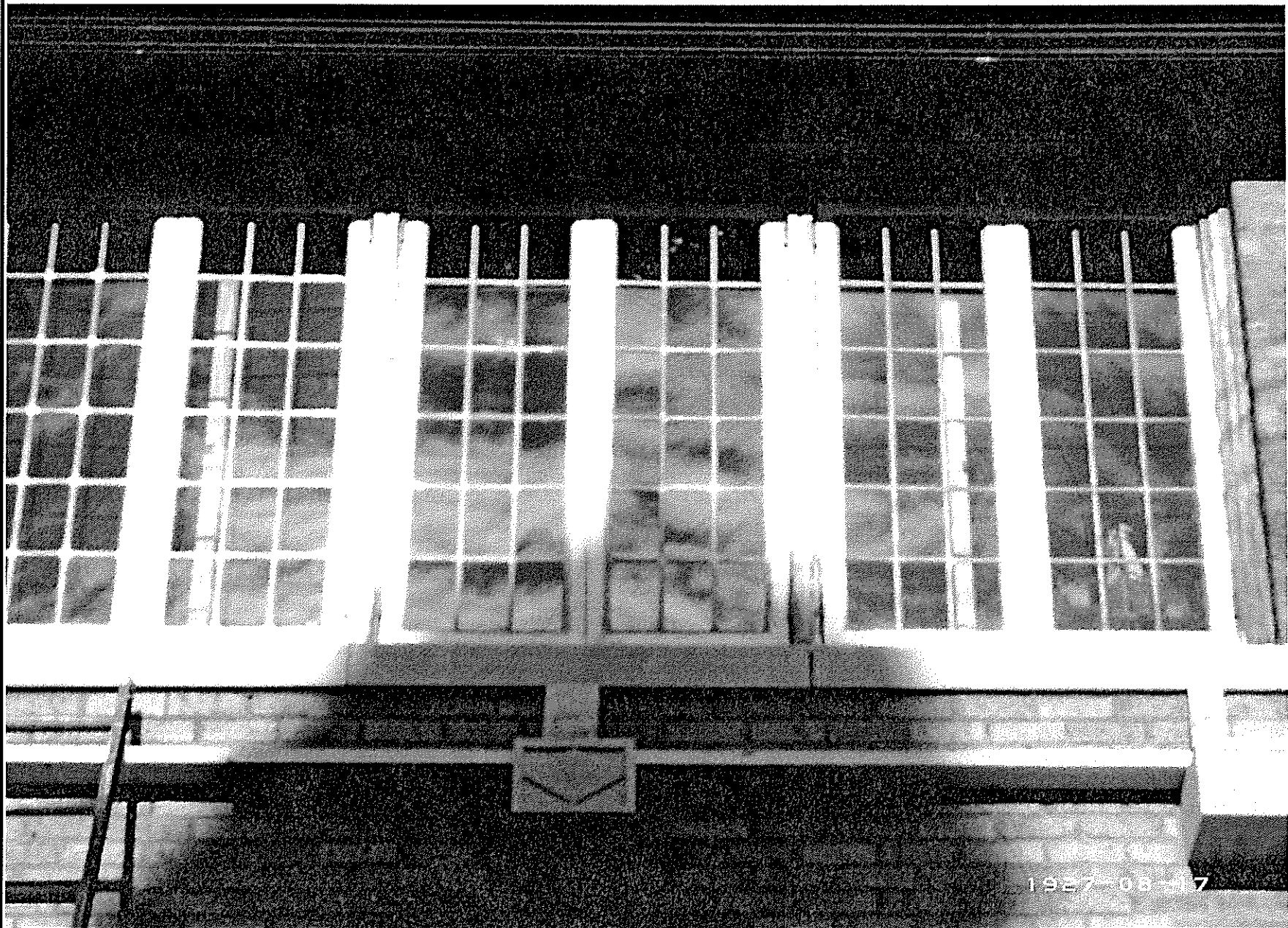
Casement windows on all three sides of second story room over garage will be restored using modern restoration techniques
