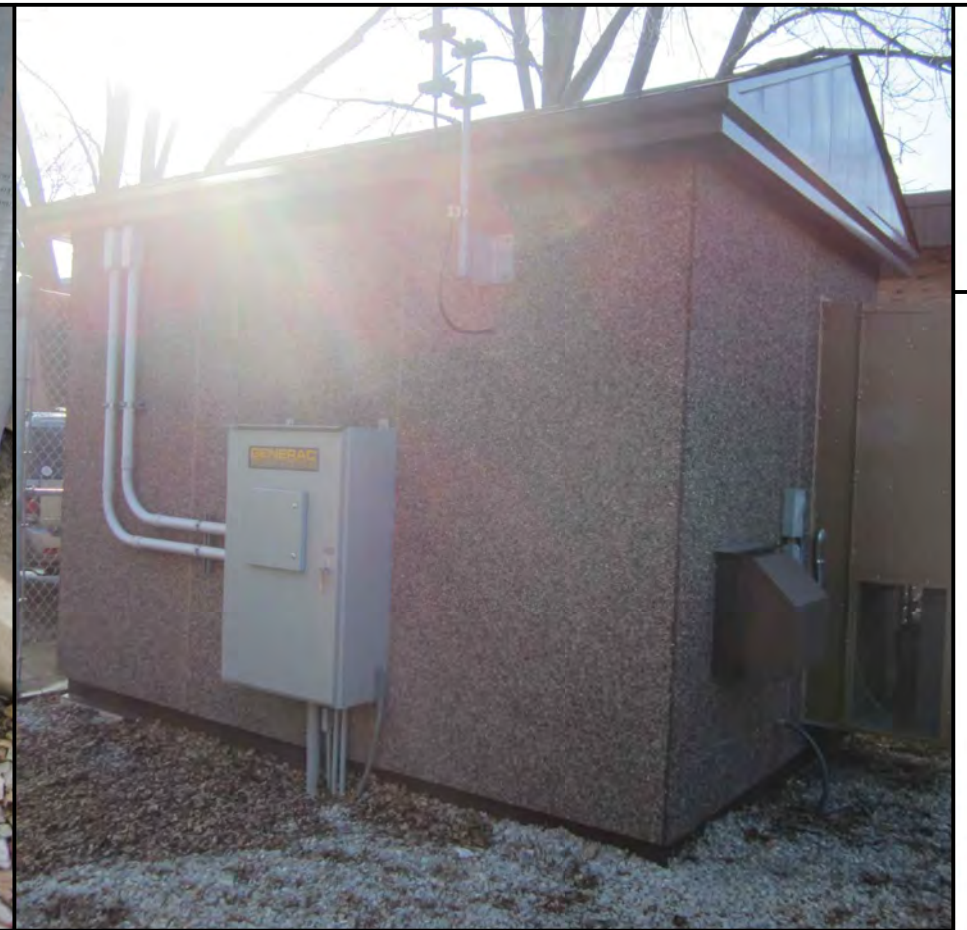
LESSEE EQUIPMENT SHELTER
