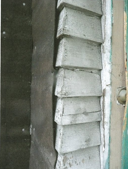
Figure 23: Corner of original clapboard siding at the front door shows salvaged wood.
