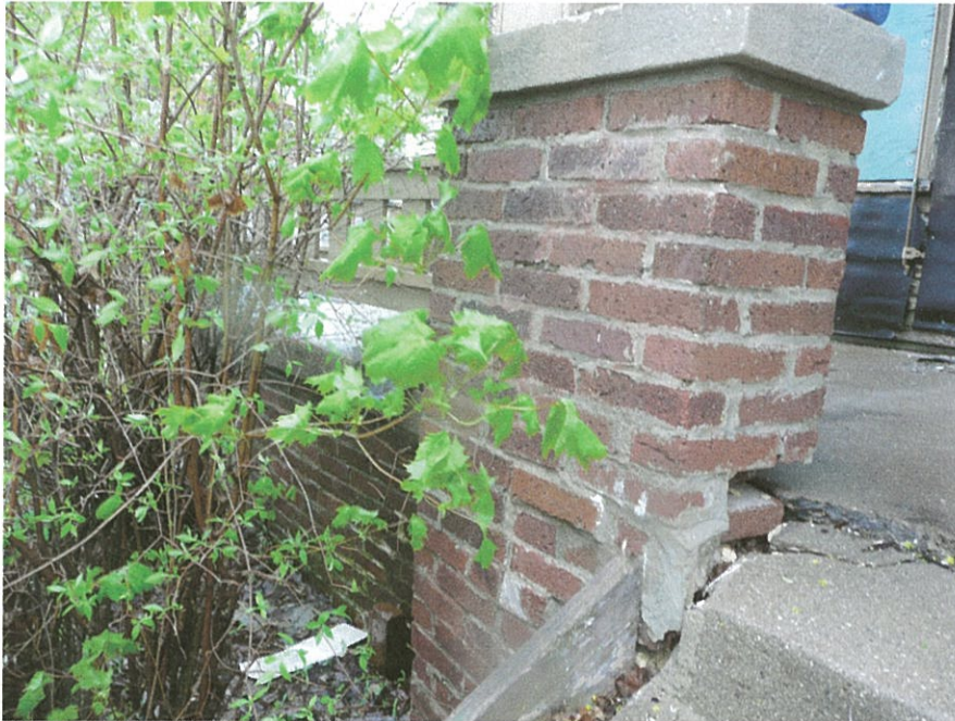
Figure 16: Shifting masonry porch piers (east elevation).
