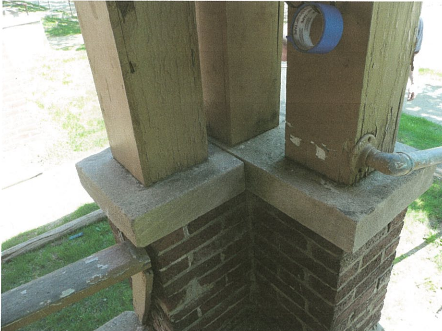
Figure 18: Wood columns supporting upper level of front porch on east elevation are original and will be restored.
