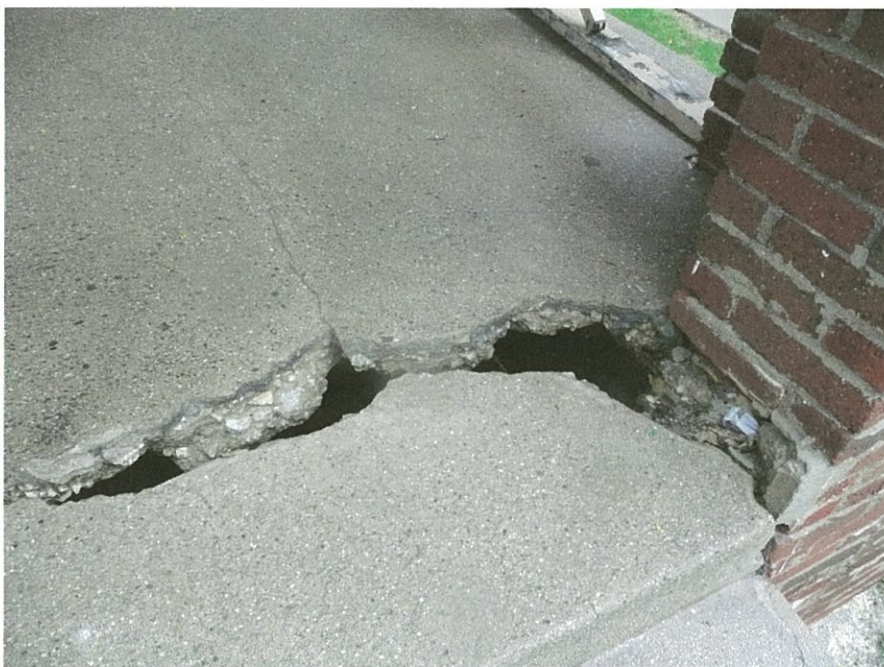
Figure 15: Cracked concrete porch (east elevation).
