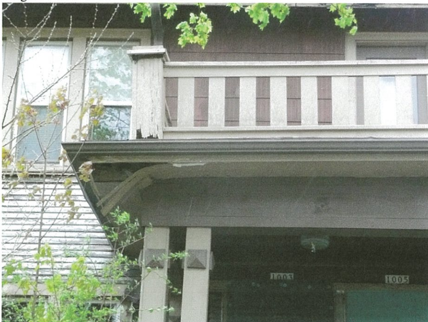
Figure 19: Detail of porch railing and tops of porch columns (east elevation). Railing is not original.
