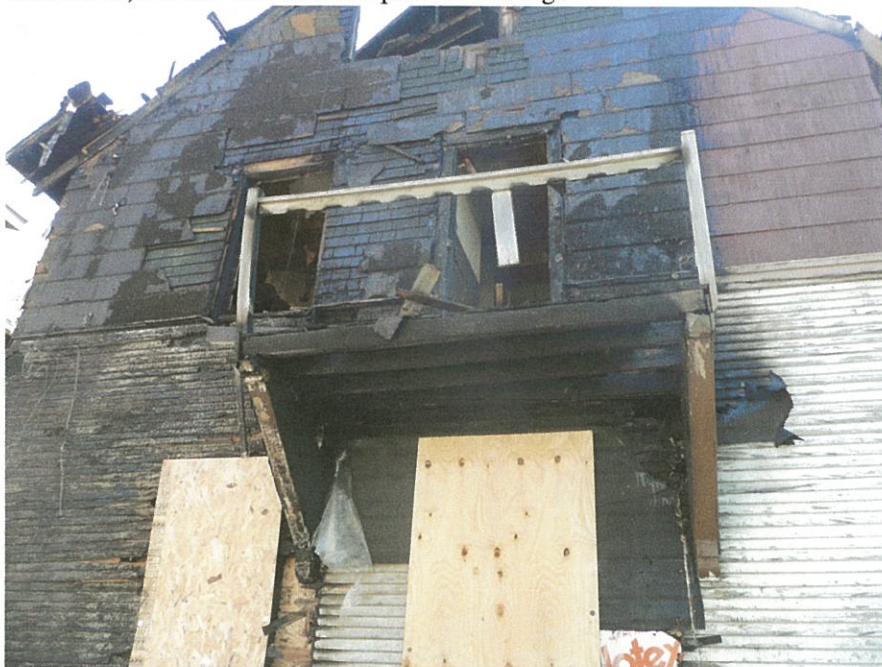
Figure 22: Airing porch following May 15 fire (west elevation). This porch structure is not salvageable.
