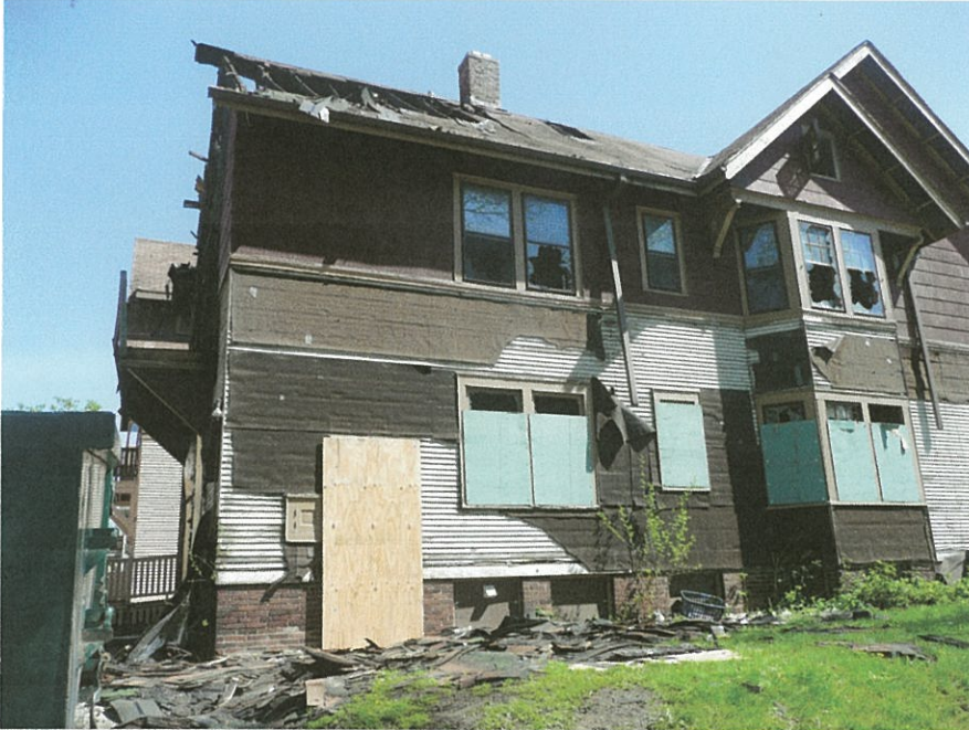
Figure 5: South elevation after May 15 fire.
