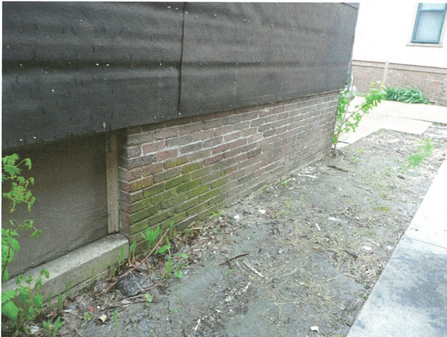
Figure 24: Algae growth on water table masonry courses.
