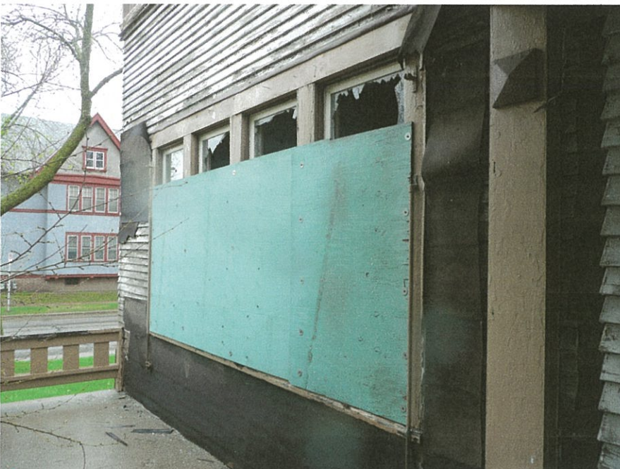
Figure 12: First floor windows boarded up following an earlier fire (east elevation). Note all glass and mullions are missing.
