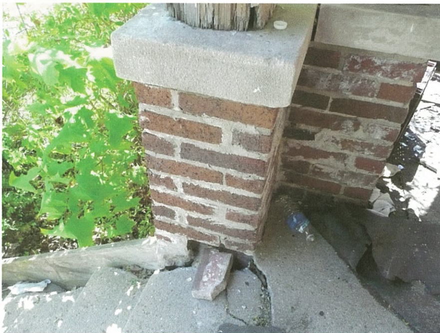
Figure 17: Mortar patching, loose brick on masonry porch piers (east elevation).
