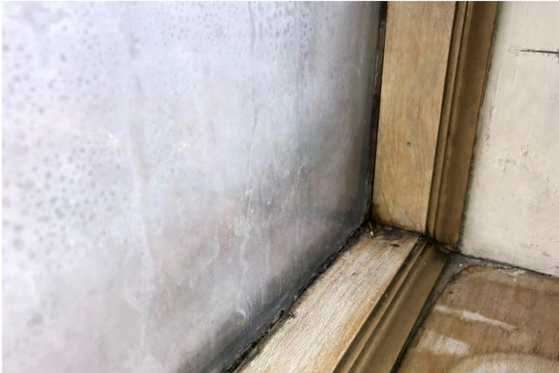
IMAGE 29: View of moisture along glass and at frame corner. Preserve, LLC 2021.
