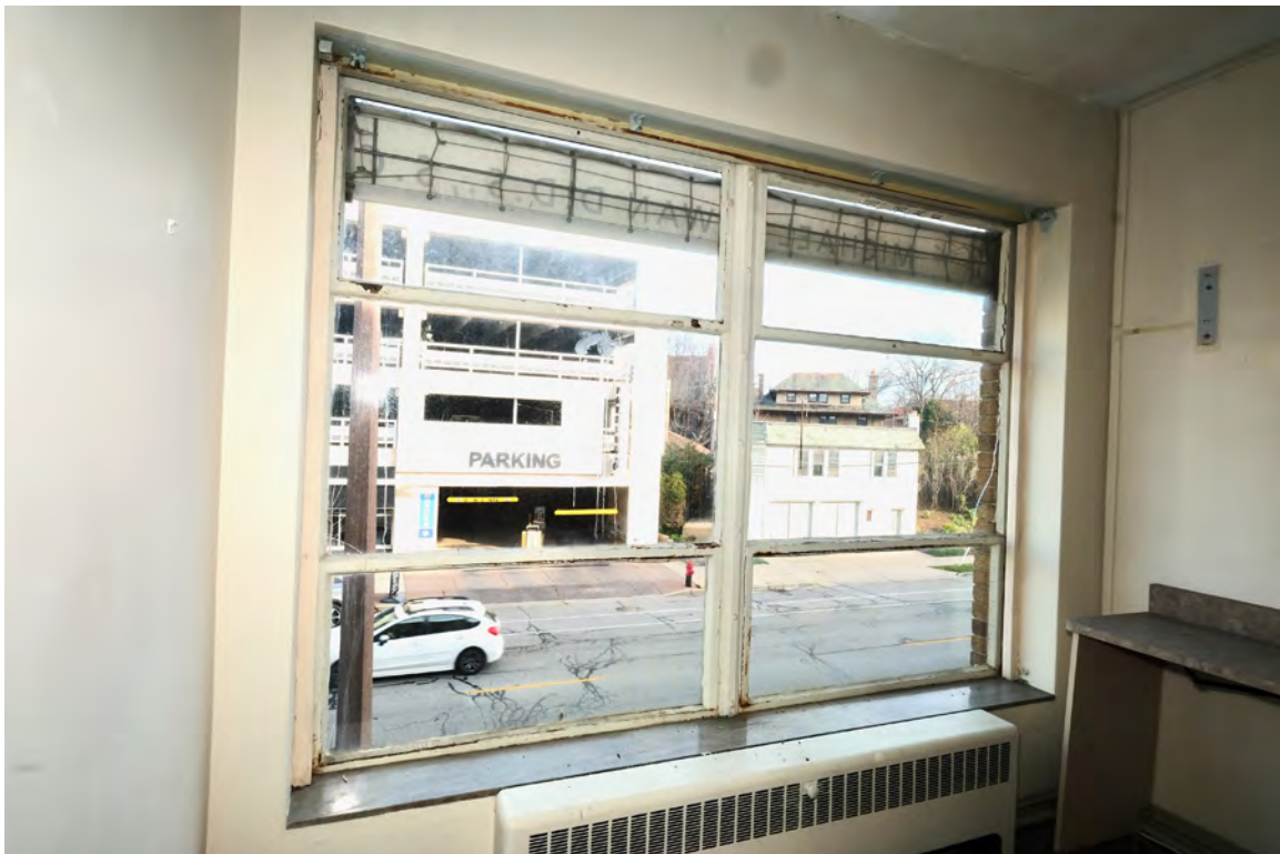
IMAGE 8: Interior side of east-elevation window units. Corrosion is evident throughout and units no longer operate. Preserve, LLC 2021.
