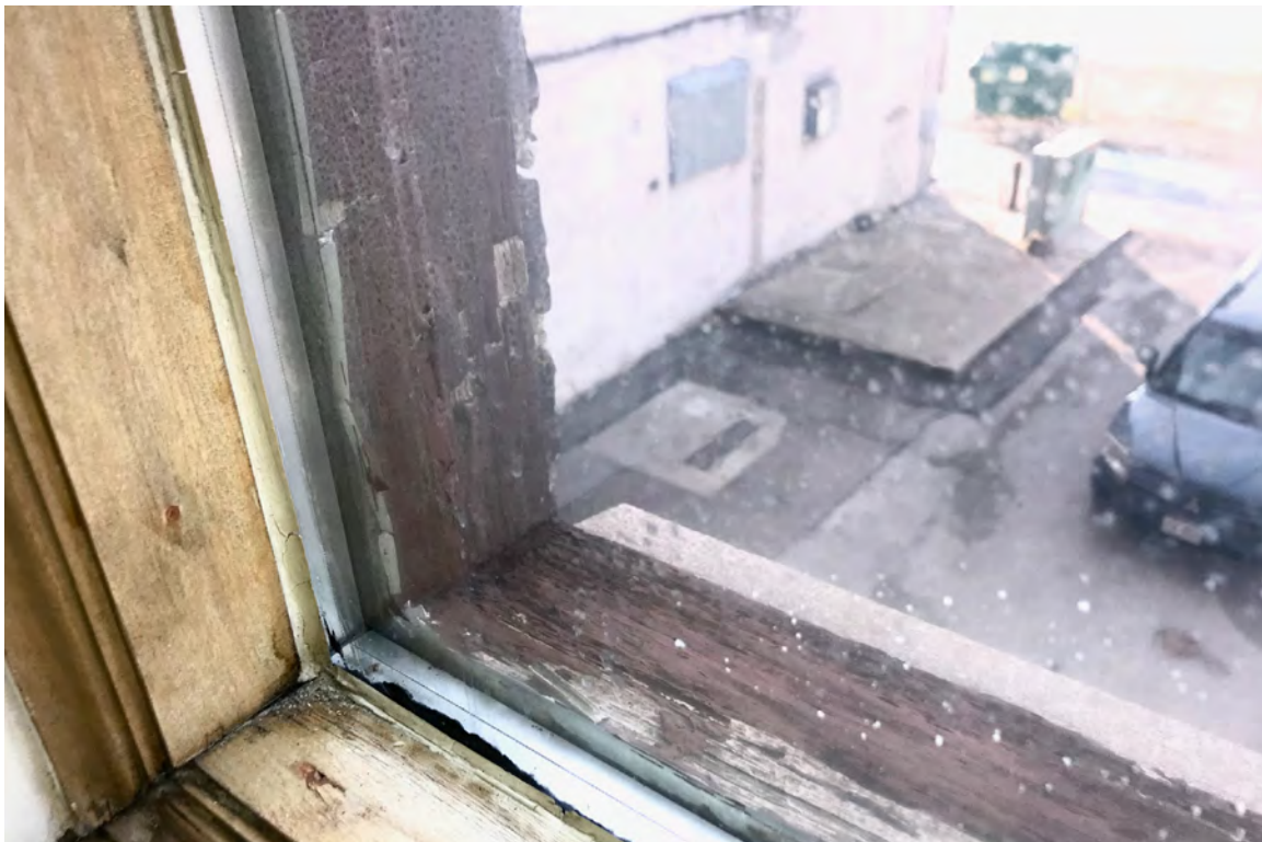
IMAGE 28: View of typical corner frame and sill conditions at a west elevation window. Preserve, LLC 2021.
