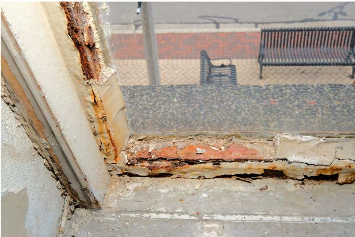
IMAGE 16: View of more severe corrosion at window unit corner. Preserve, LLC 2021.
