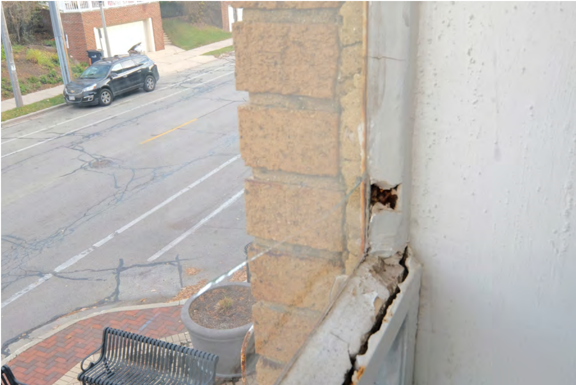
IMAGE 15: View of frame and sash separating at window. Preserve, LLC 2021.
