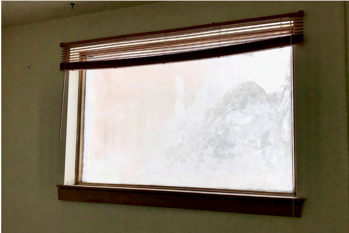
IMAGE 25: View of typical west-elevation window unit. Thermal pane seals are broken and windows leak, resulting in frost and ice forming between the panes. Preserve, LLC 2021.
