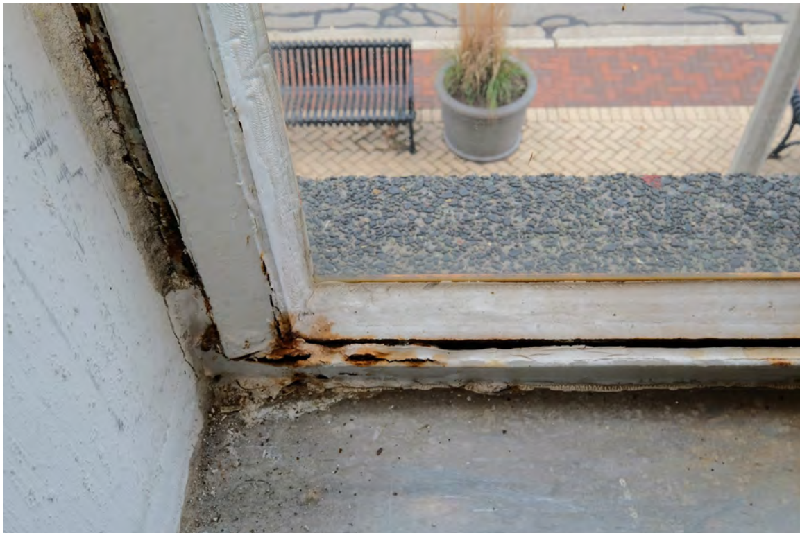
IMAGE 14: View of typical corrosion at frame corners. Frame members and sashes have moved out of plumb due to jacking. Preserve, LLC 2021.
