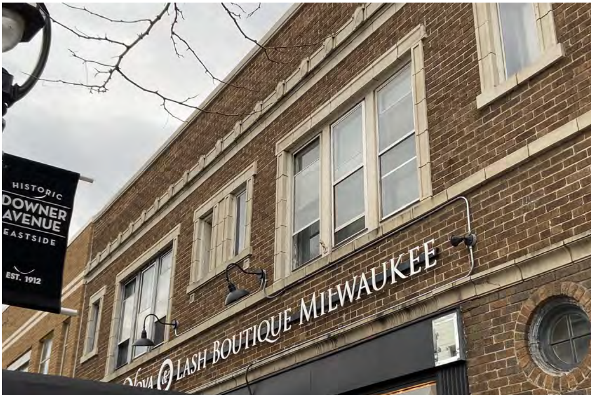
IMAGE 32: View of windows to be replaced on the second floor of the Downer Theater. Preserve, LLC 2021.
