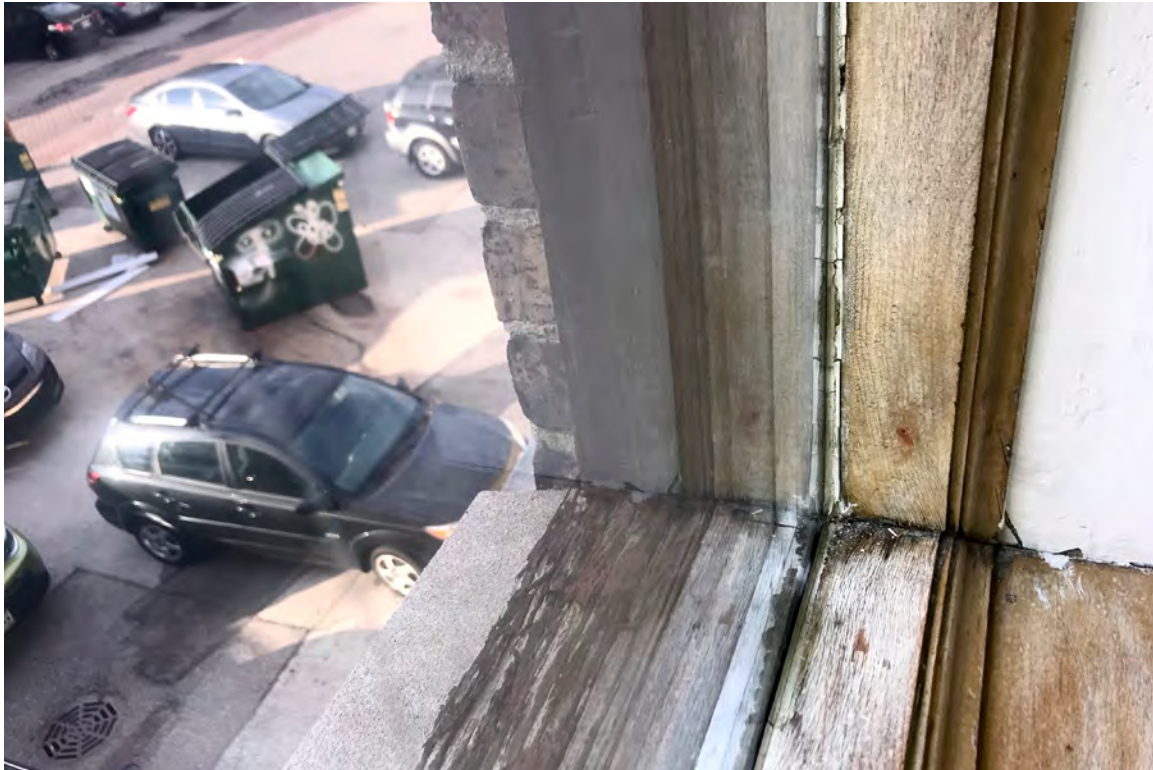
IMAGE 27: View of the typical corner frame and sill at a west elevation window. Seals are broken, wood is rotting, and the exterior sill is almost completely deteriorated. Preserve, LLC 2021.
