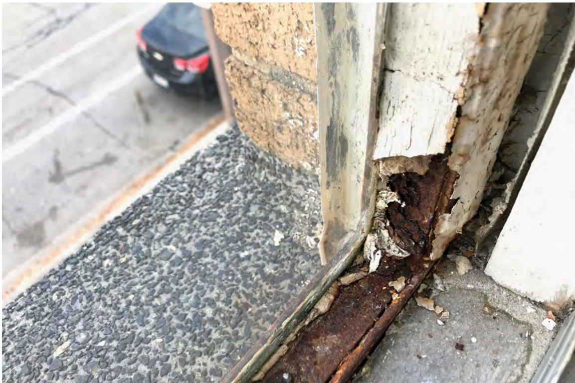
IMAGE 20: View of severe corrosion at the corner of a second floor window frame. Preserve, LLC 2021.
