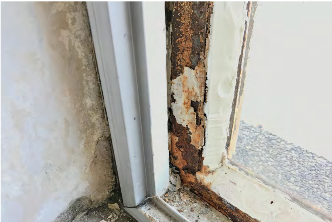
IMAGE 18: View of heavily deteriorated and corroded corner of window frame. Preserve, LLC 2021.
