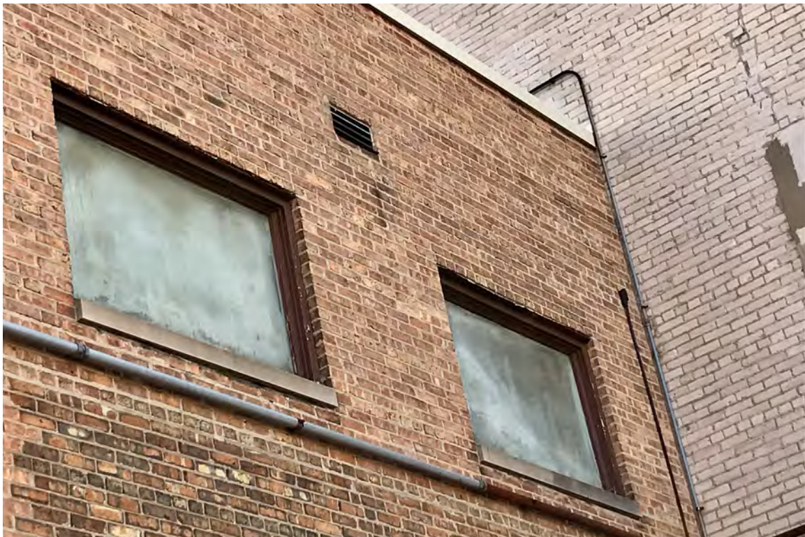
IMAGE 22: View of units with frost and ice located between the panes. Preserve, LLC 2021.
