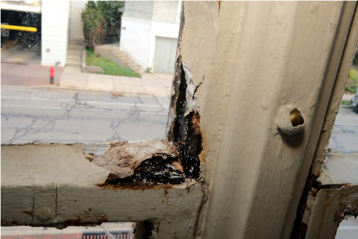
IMAGE 17: View of more severe corrosion at operable sash corner. Preserve, LLC 2021.
