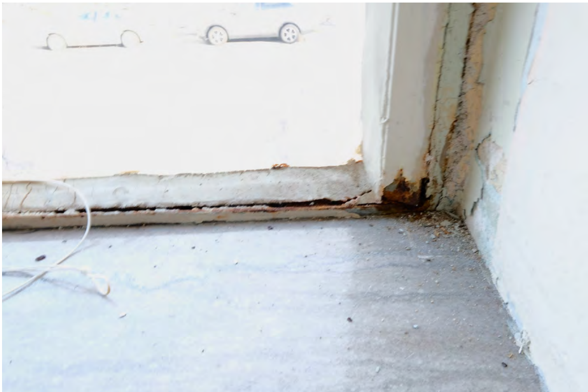
IMAGE 6: Typical corrosion location at the frame corners. Also note expansion cracks at frame and cracked sealant. Preserve, LLC 2021.
