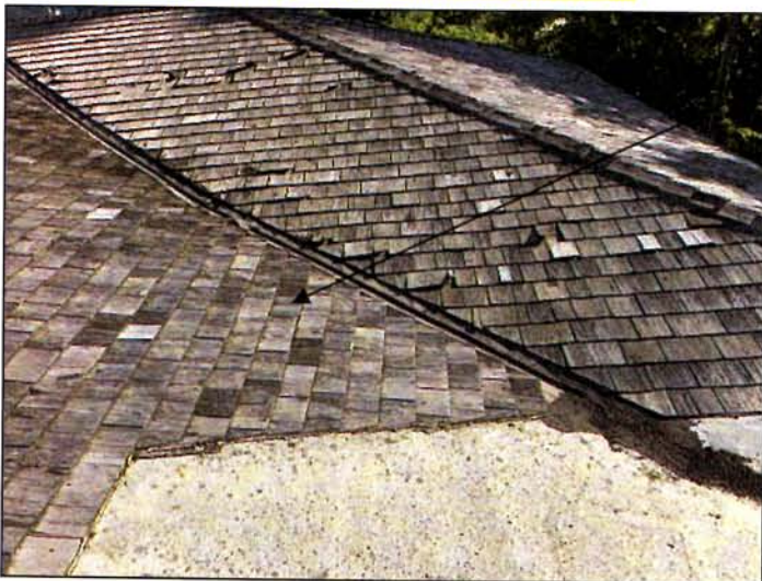
On both sides on the rear, the new membrane will extend all the way into the valley to help prevent undesired penetrations
