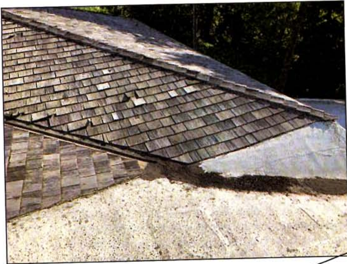
Actual knots in the wood throughout the entire roof
