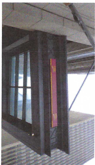
Existing 8" h x 6'-0" w sign to be removed & replaced. Wall patched and painted as required.
