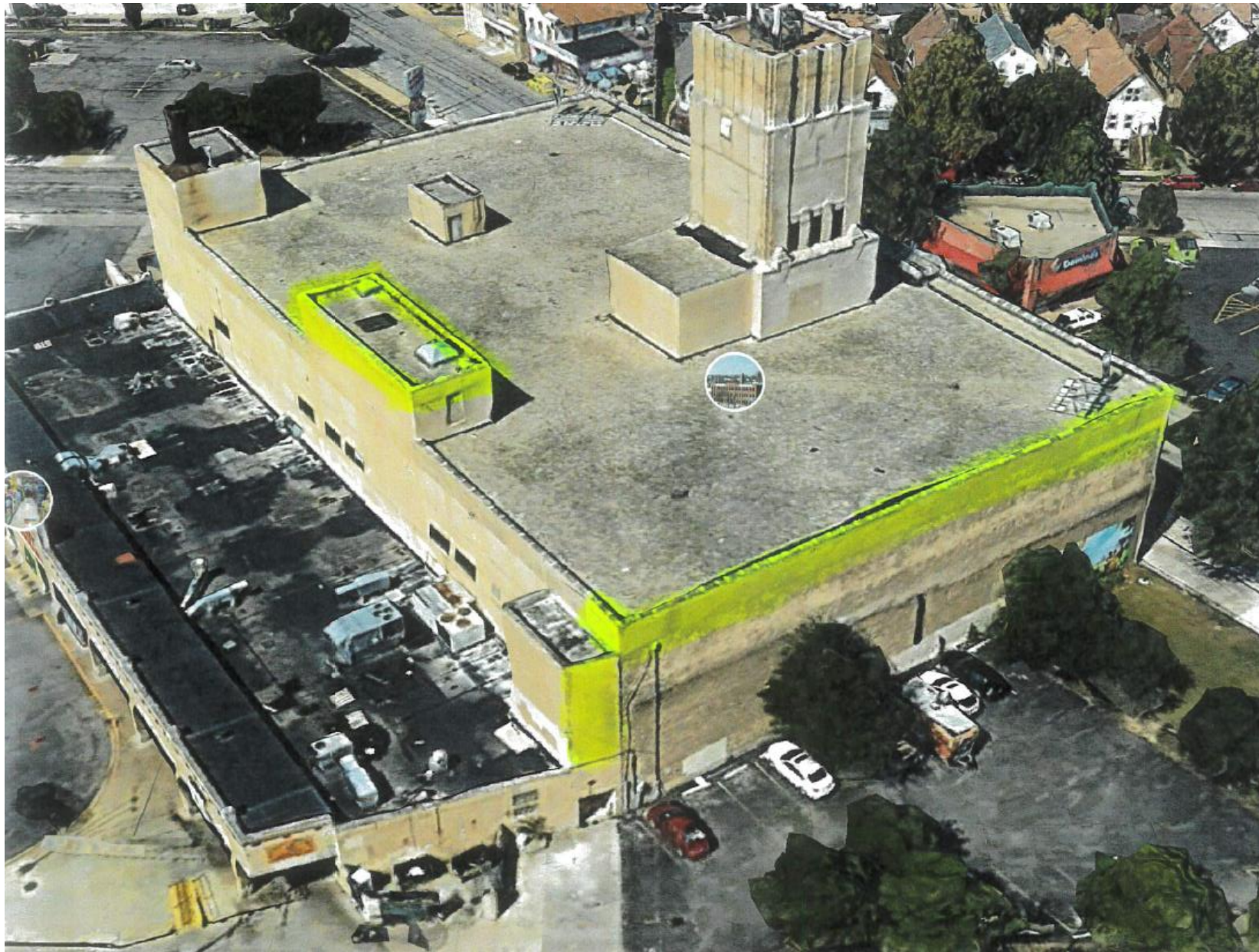
Highlighted areas to be reconstructed in-kind
