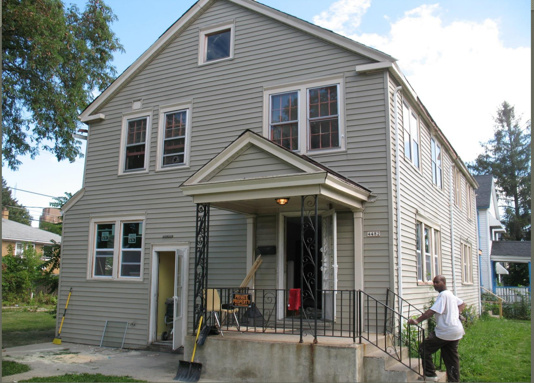
Photo by Carlen Hatala during work in progress. Main windows appear readily repairable.
