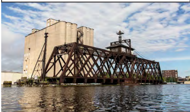
Unused railroad swing bridge in the Milwaukee River near Florida Street. photo by Eddee Daniel
