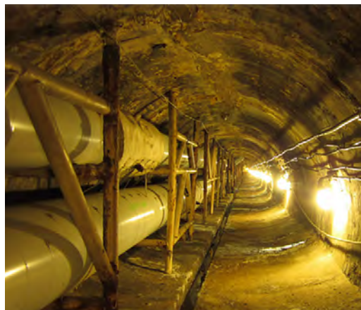
Pipes carrying steam from the Menomonee Valley Power Plant to customers in the downtown area.
