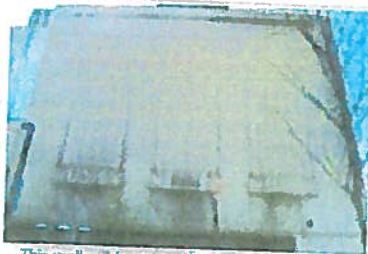
This wall will be moved 39 feet into N. 2nd St. Photo by Brian Jacobson.
