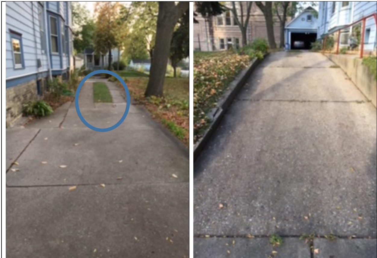
Photo at left shows section of driveway closest to the garage and the center section (circled), which will be replaced. Photo at right shows section of driveway closest to N. 31 st St. Retaining walls along this portion of driveway will not be affected.
