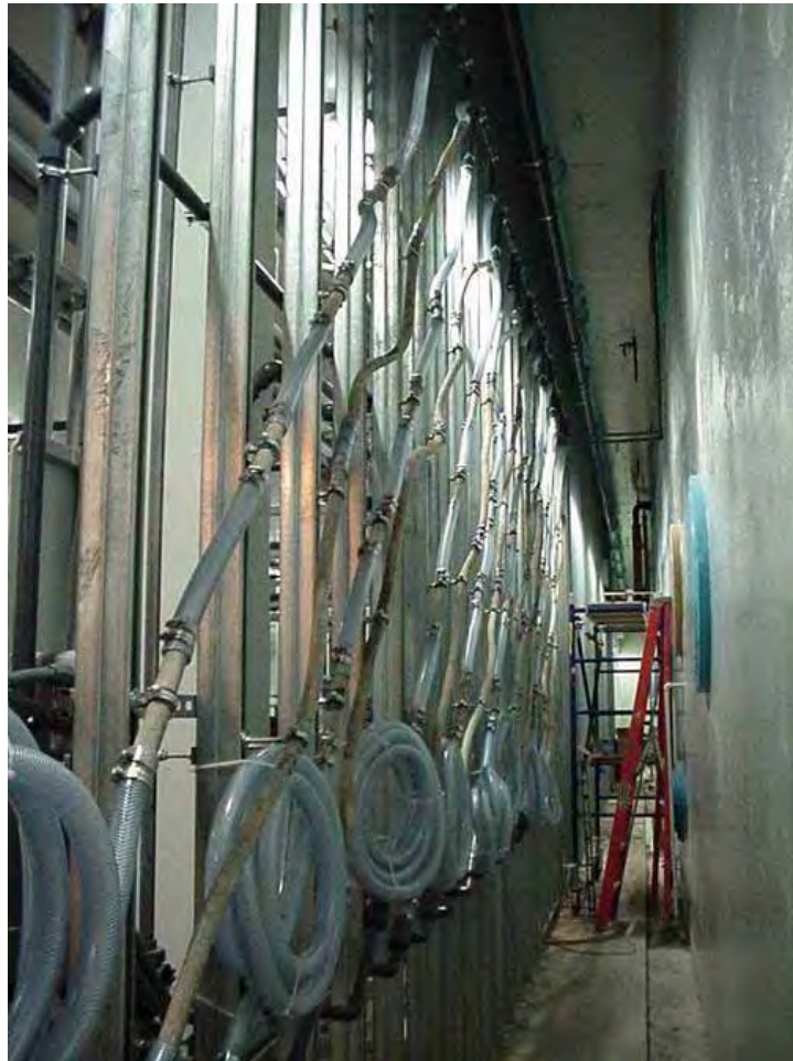
Figure C.87 Photograph of Washington Aqueduct Pipe Rack
