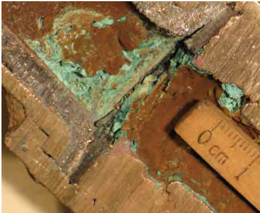
Figure F.46 Photograph of Pipe PX09 from Site D-2
