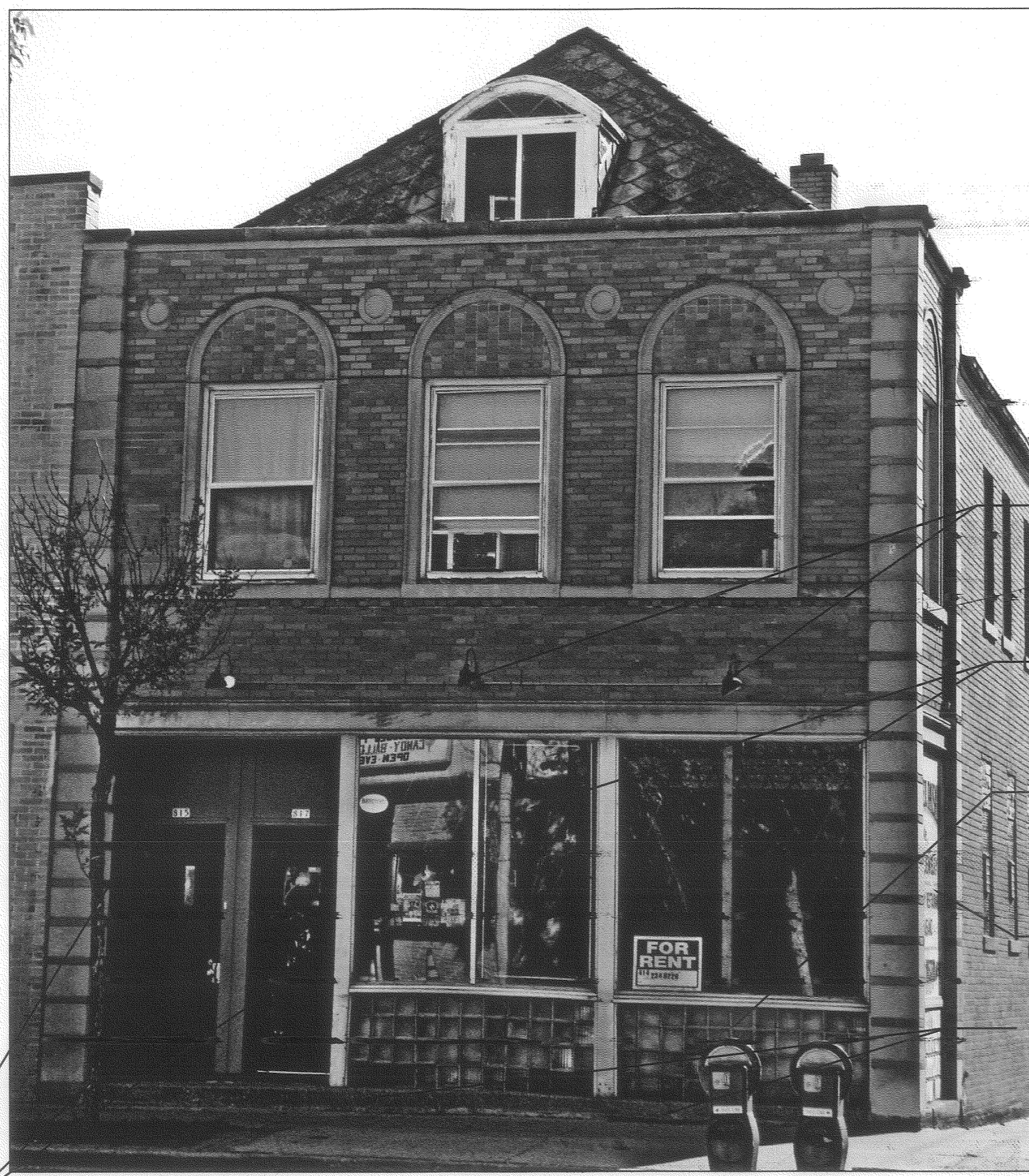
1 REMOVE EXISTING DOORS REMOVE EXISTING TRANSOM PANELS ABOVE BOTH DOORS EXISTING NORTH ELEVATION SCALE: NTS
