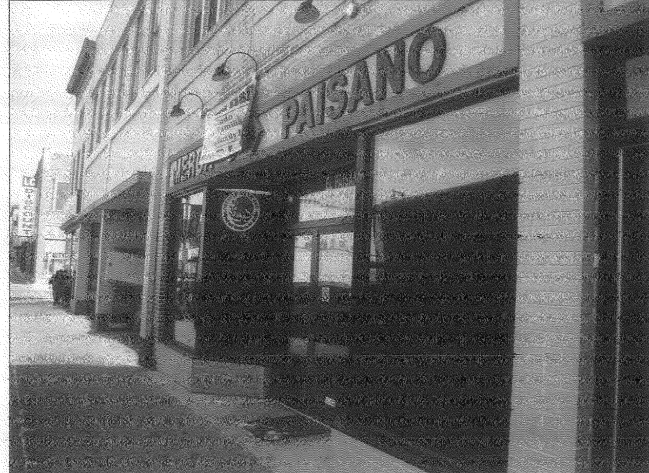
3 EXAMPLE OF EXISTING ALUMINUM FRAMING; STOREFRONT; DOORS; FRAMES AND TANSOM AND GLAZING. THIS IS TO BE MATCHED AT 815-817 ADDRESS EXISTING ELEVATION - EXAMPLE SCALE: NTS
