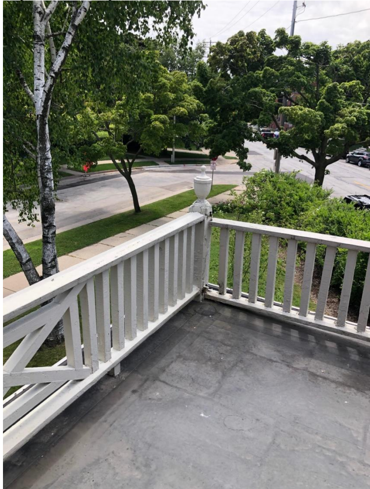
South balcony showing one of the damaged posts.
