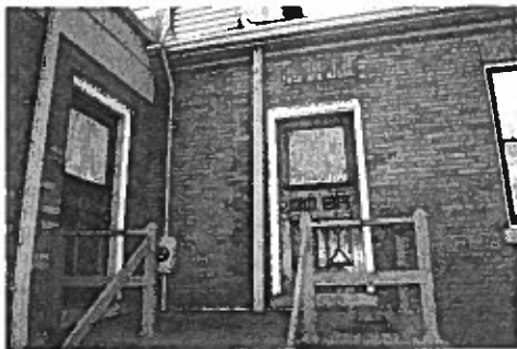
Figs. 14-16 Side Doors, Details showing damage from weather exposure.
