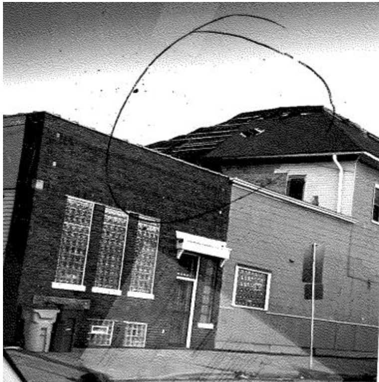
Fire damage is primarily on the north side of the hipped roof.
