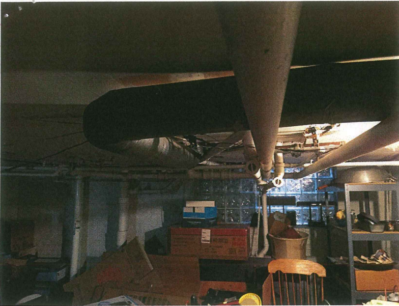
Existing Ductwork for Downdraft Range
