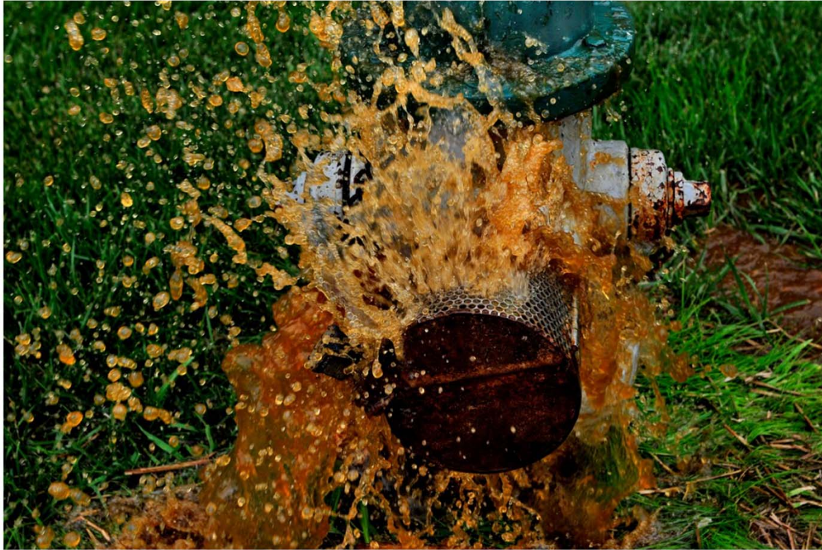
Brown water pours from an opened hydrant on Wednesday in Potomac, Md. Montgomery County residents have been making reports about it since March. Officials blame salt and manganese. (Michael S. Williamson/The Washington Post)
