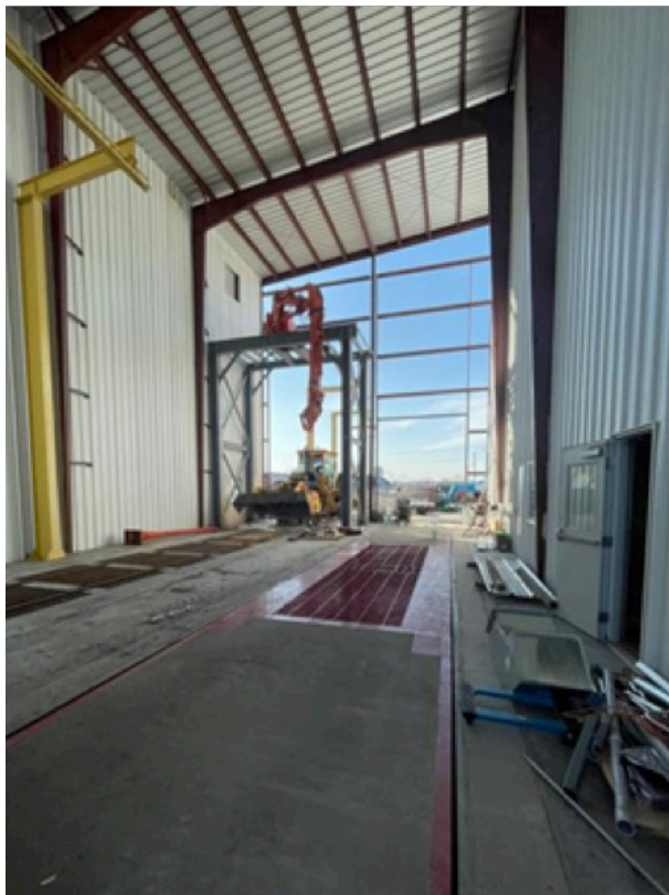
Figure 8: Receiving Building with Truck and Rail, Hard Car Unloader, and Fall Protection
