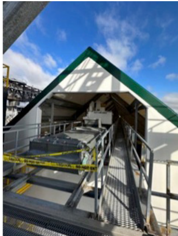
Figure 9: Grain Vessel Loader and Grain Handling Equipment
