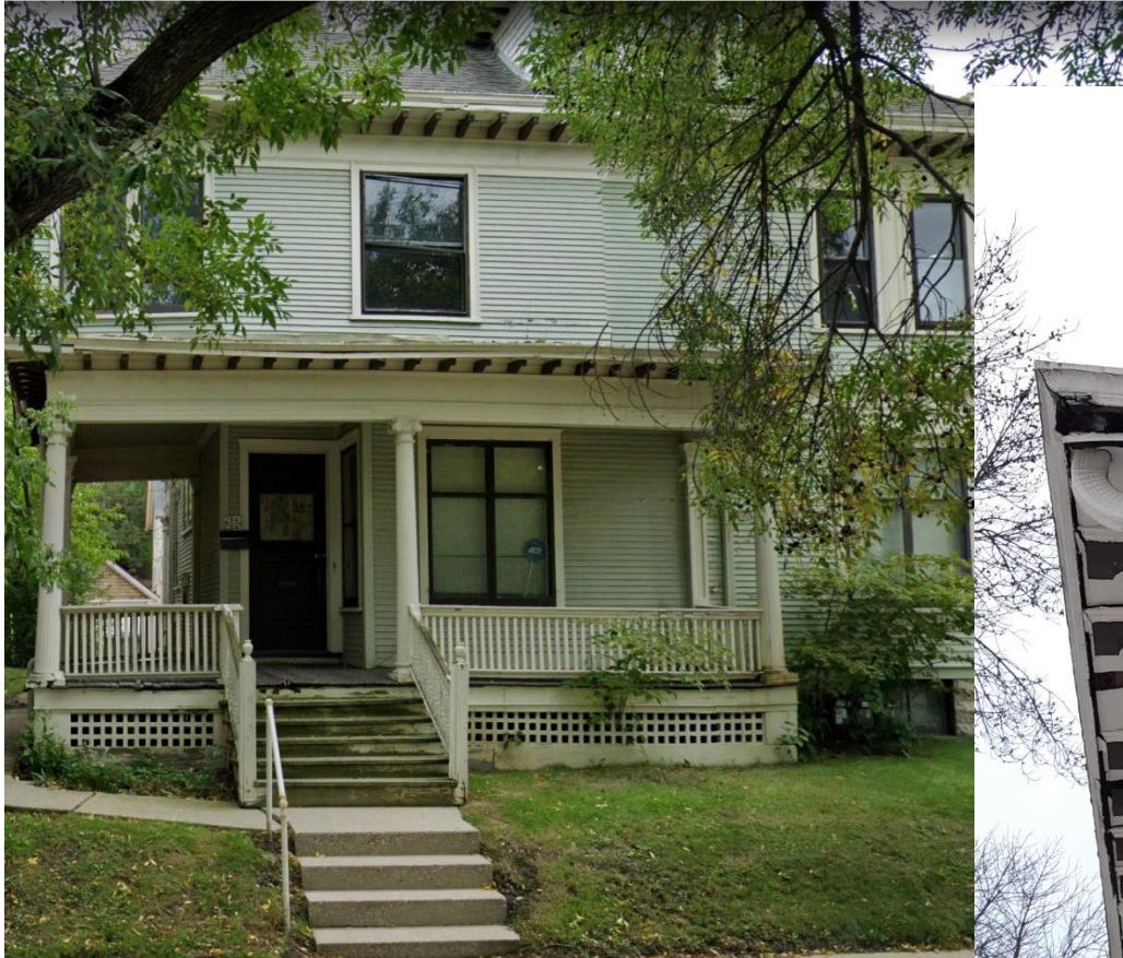
Downspouts and wooden gutters to be replaced
