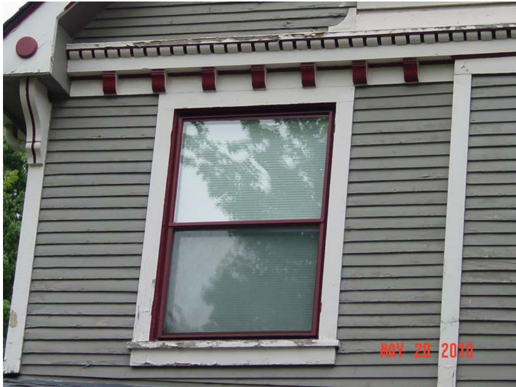
Example of some peeling and flaking of paint on front elevation
