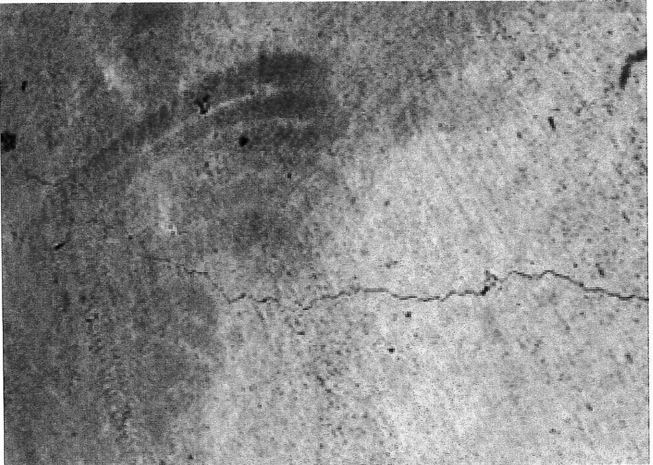
Close up of the Crack
