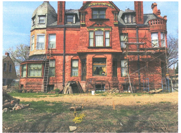
East side middle of the mansion, big window in the middle, door to outside is on the left. Porch will go from where the ladder is to the door.
