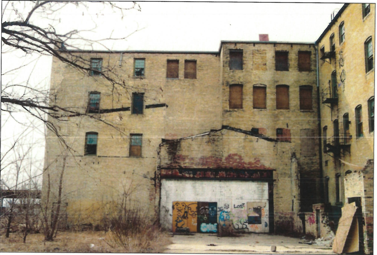
Wisconsin Historic Preservation Database, 2018 photograph (WHPD #110095) East elevation – appearance of the building when National Register-listed in 2018
