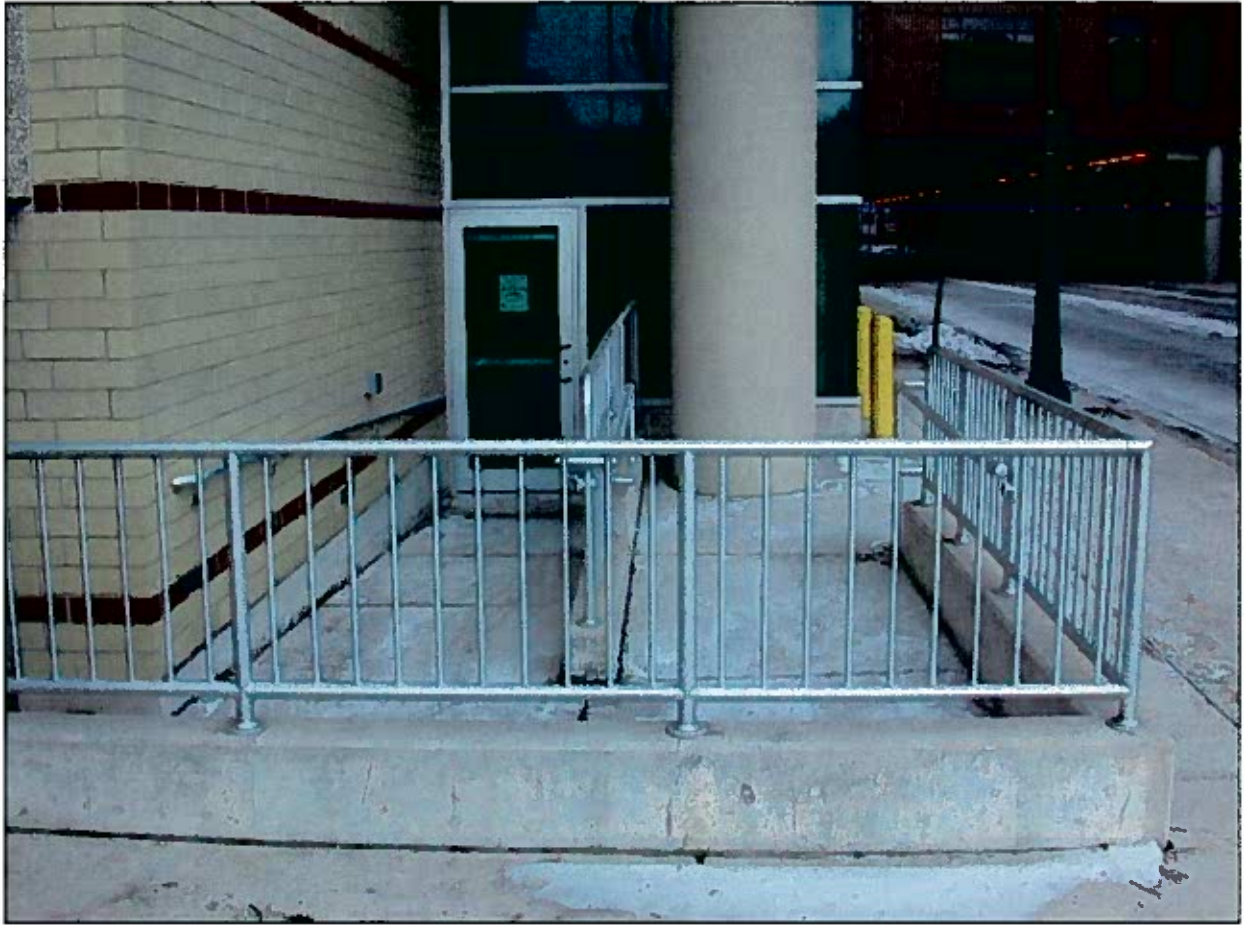
3001 North 51st St. 071000 1-31-08 Looking North from the west side of North 51st Street at the pedestrian ramp
