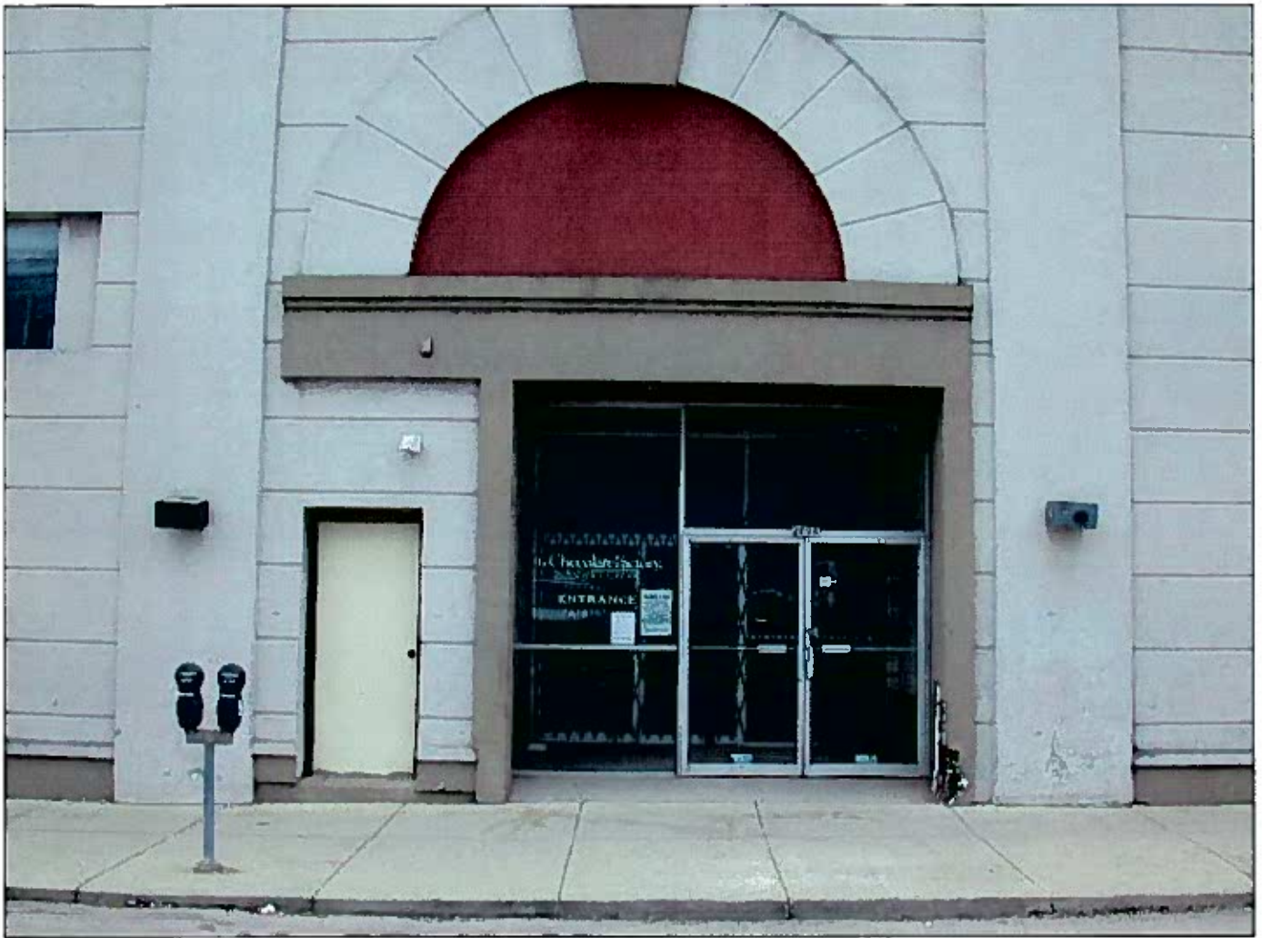
2217-39 North Prospect Ave. 071654 05/01/08 Looking southerly at the non-code compliant hood on the south side of East Ivanhoe Place
