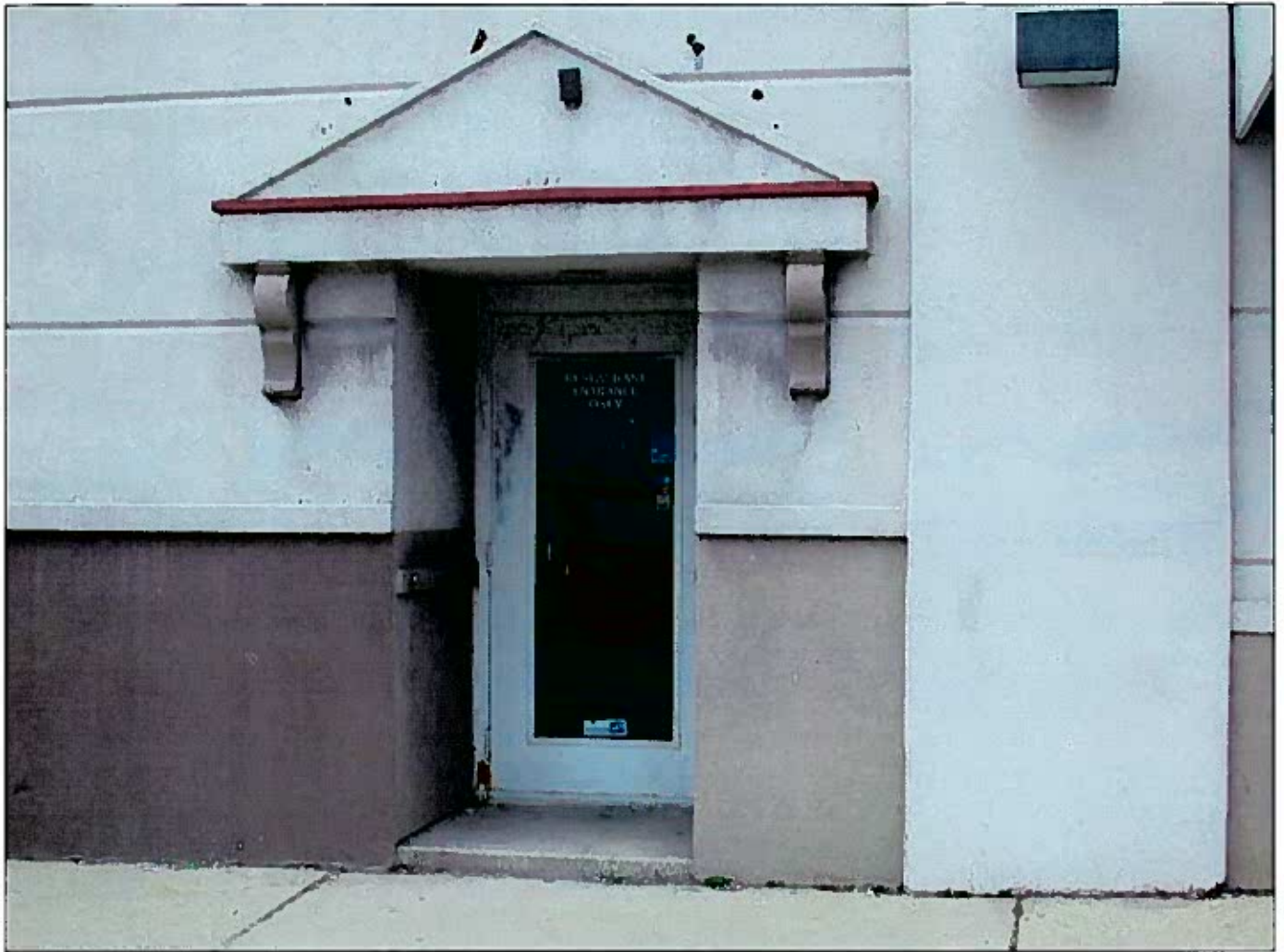
2217-39 North Prospect Ave. 071654 05/01/08 Looking northwesterly at the non-code compliant hood on the west side of North Prospect Avenue
