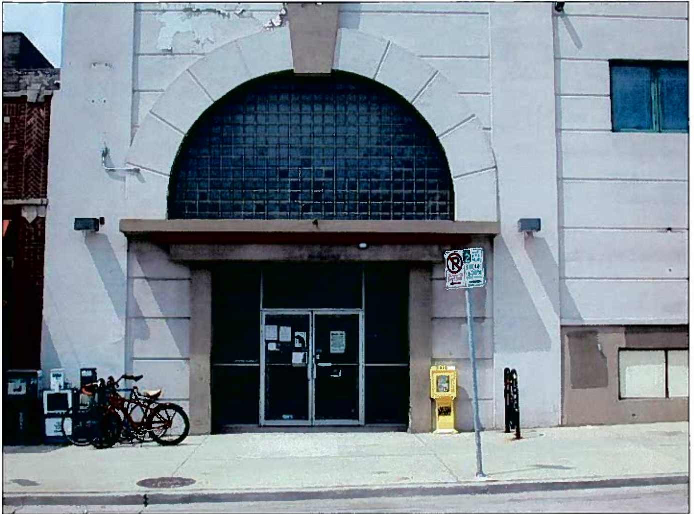
2217-39 North Prospect Ave. 071654 05/01/08 Looking northwesterly at the entrance and non-code compliant hood on the west side of North Prospect Avenue
