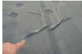
Roof 1 w/ membrane bulges
