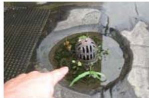
Roof 2 w/ vegetation growth
