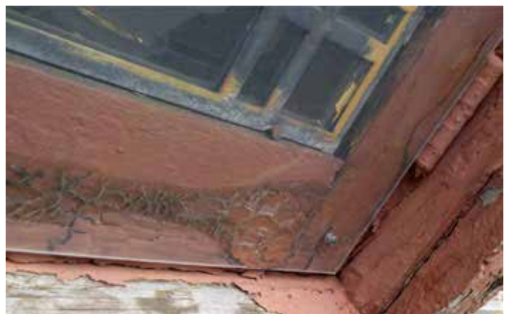
Lead paint chipping from a window.
