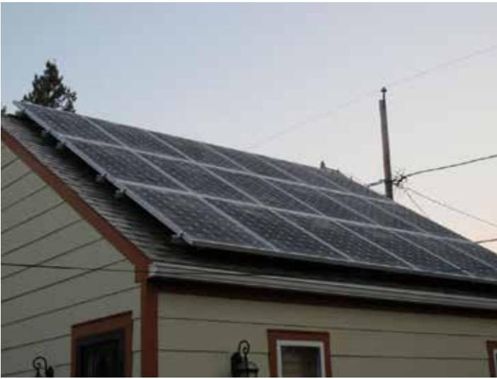
Example of rooftop solar.
