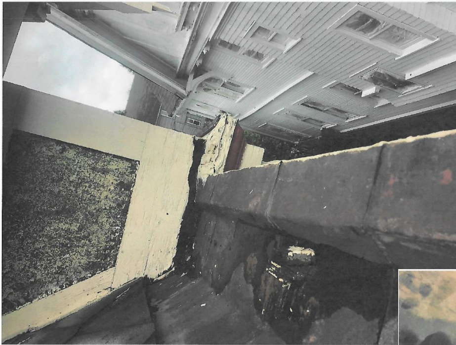
Typical gutter and wood decay conditions
