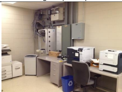
City Communications Equipment
