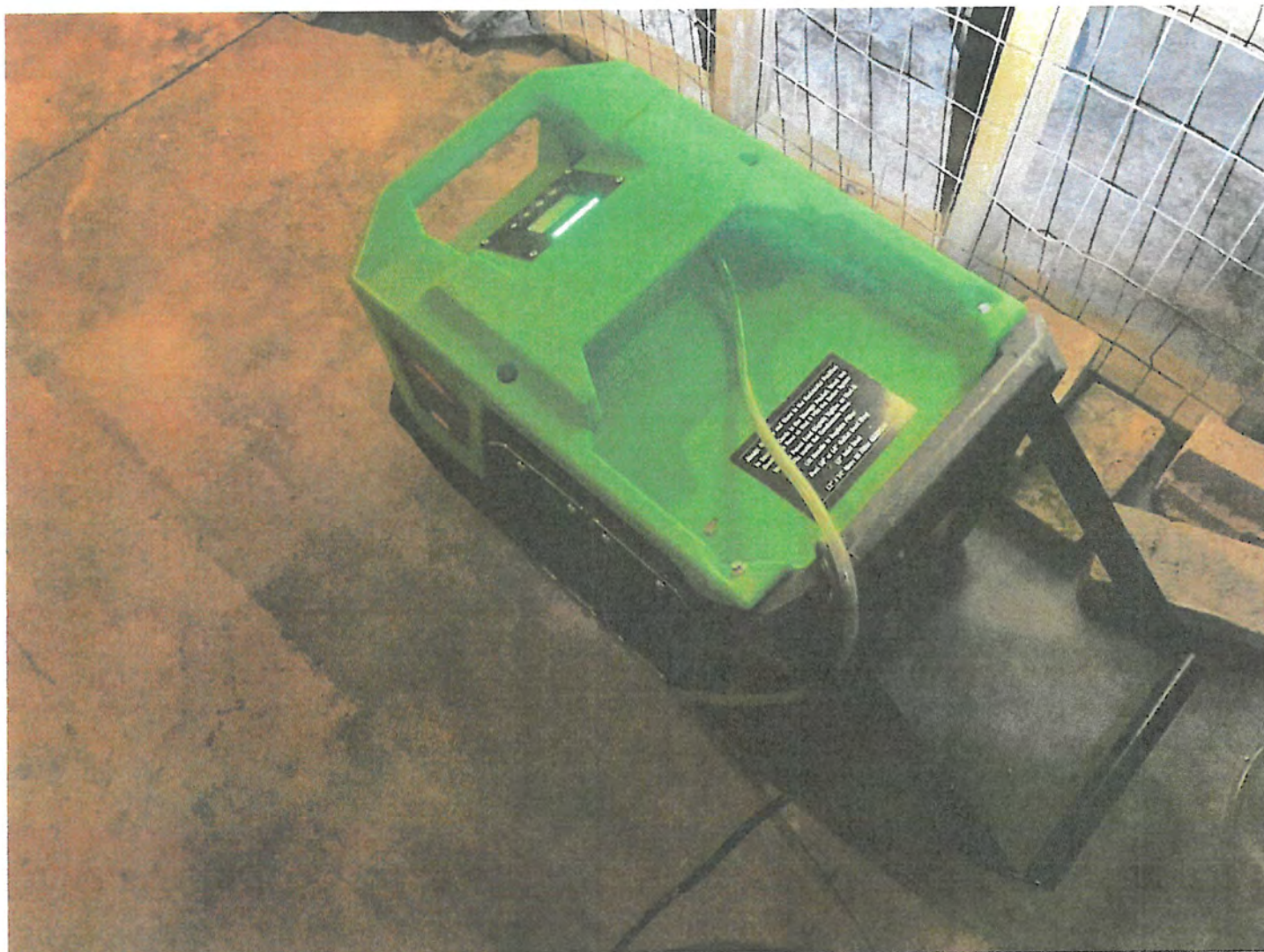
15 15-1 more dehu in Basement on 7_ Date Taken: 7/25/2025 25, placed on 7_
