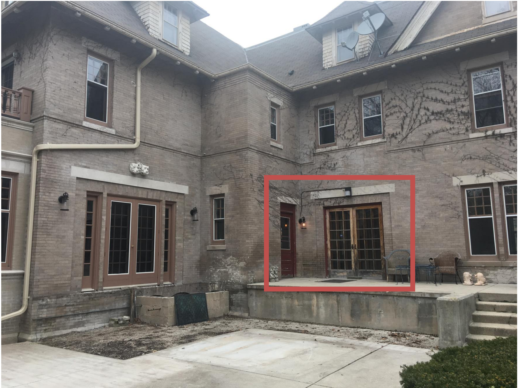
Expanded rear view. Highlighted screen doors to be replaced. Metal security doors shall match the grid pattern of the highlighted French doors.
