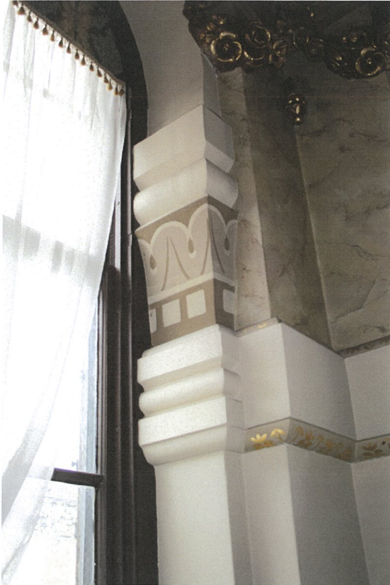
Photo No. 63: Window opening revised to access stair exit - Side wall details to be protected
