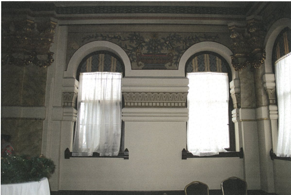
Photo No. 60: Level 2 View south gridline 10 window opening and sill cut down to access stair exit
