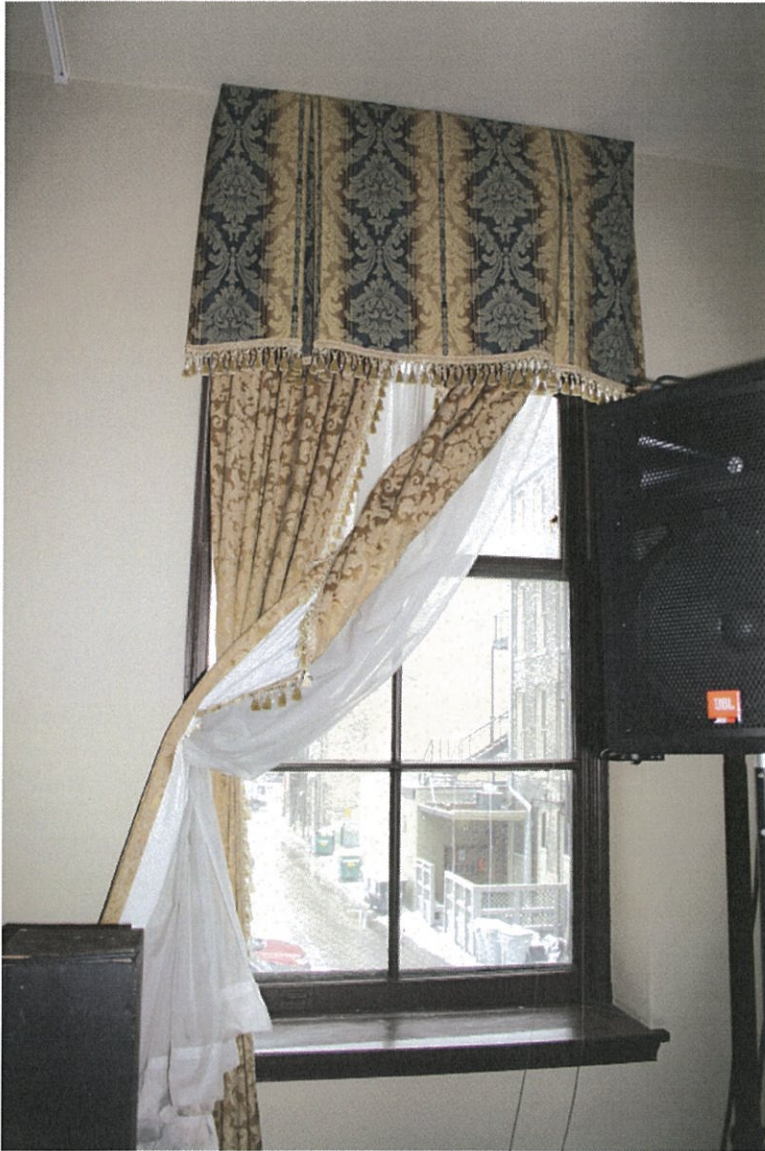
Photo No. 58: Level 1 southwest view of window - access to new stair addition - gridline A & 10
