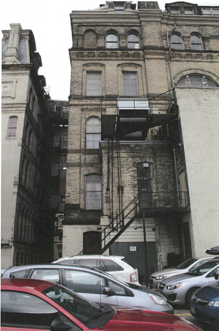
Photo No. 53: South facade location of new structure engulfing addition and three historic windows
