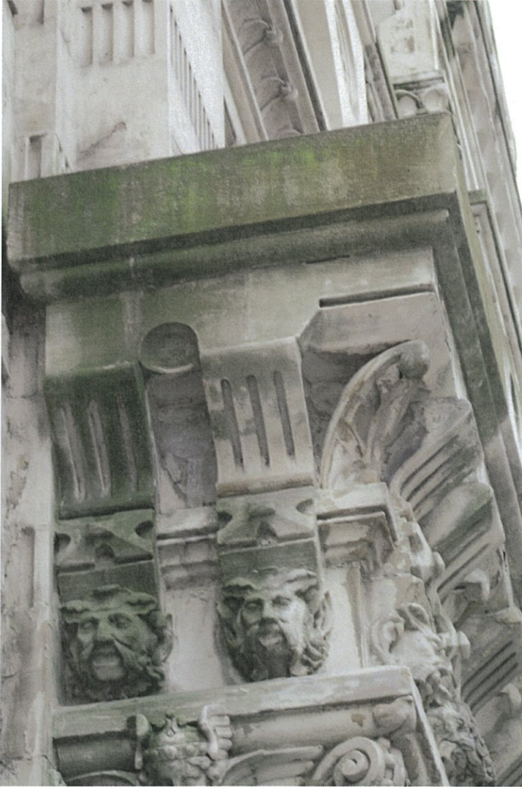
Photo No. 49: Algae built-up along entire Entablature over entry door
