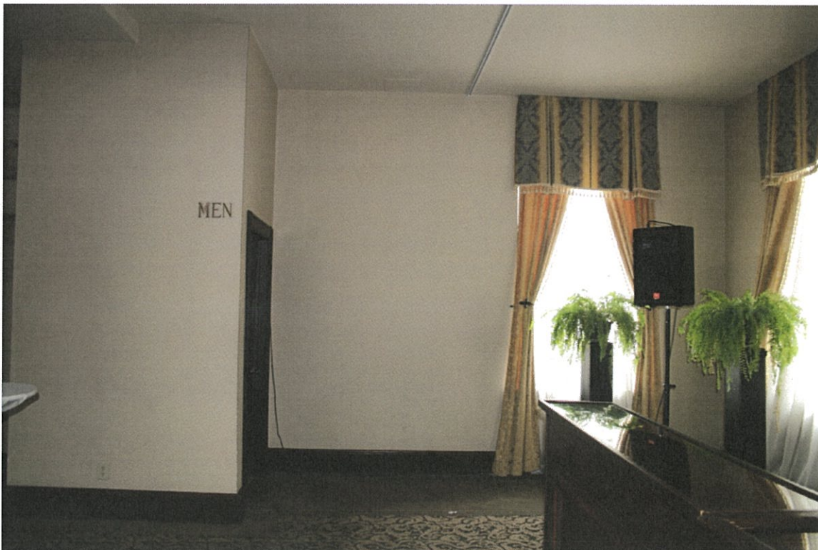
Photo No. 57: Level 1 southwest view gridline A & 10 - Window becomes opening to new stair exit
