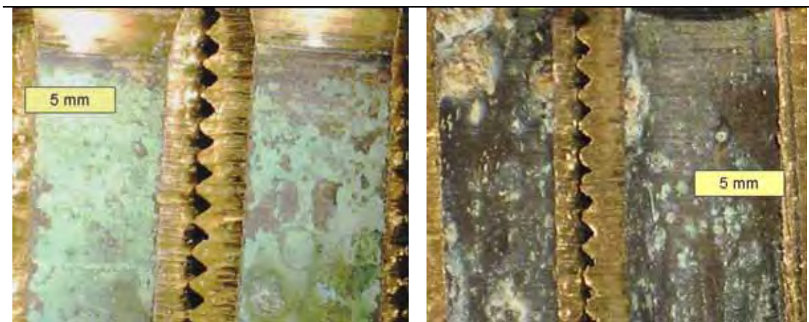
Figure F.128 Brass Supply Tubes for Faucet 08_FB02 (Site F.1). The cold water supply (left) and hot water supply (right)
