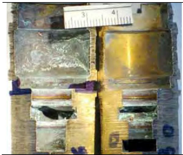
Figure F.127 Macro photograph of Interior Surfaces of Faucets at Site F1 (left) and F2 (right)
