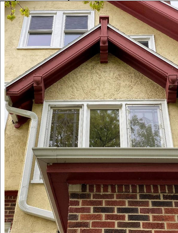
Photo showing current color of mortar and stucco.
