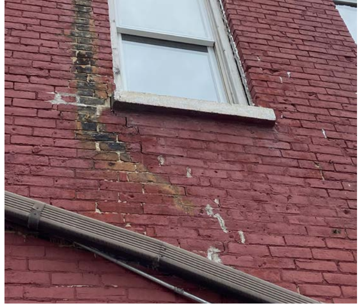
IMAGE 10: Area to be rebuilt below center second-floor window at the west elevation; large step crack and exposure to moisture has resulted in dislodged brick.
