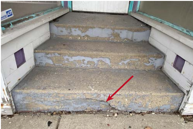
IMAGE 2: Crack at main entrance steps.
