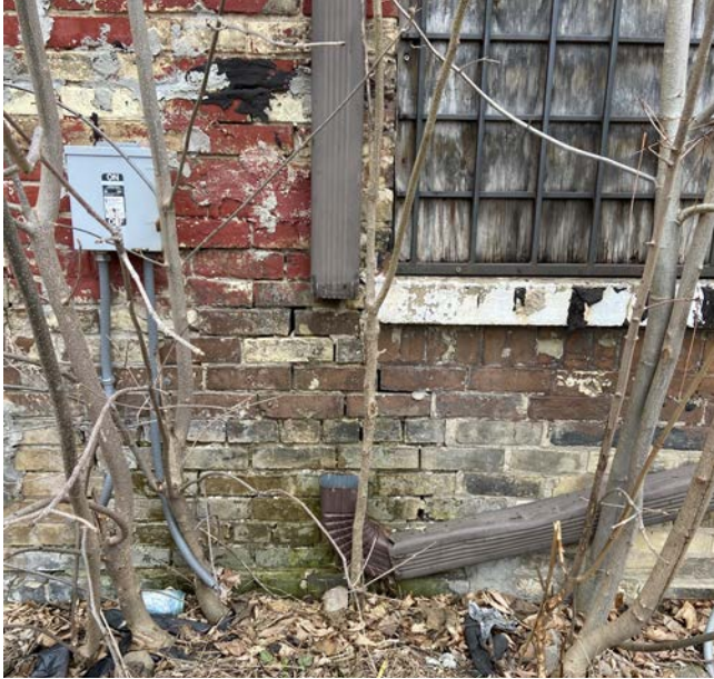
IMAGE 9: Disconnected downspouts and insufficient slope to drainage at rear west elevation near first-floor windows.
