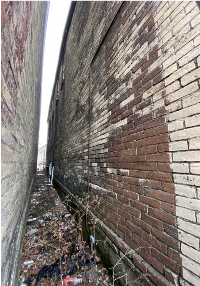
IMAGE 14: South elevation; here work is limited to masonry repairs and flashing at windows as described in the Scope Narrative.
