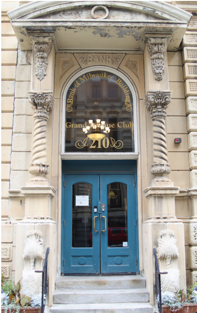
IMAGE 1: 210 E. Michigan St. entry doors, showing the existing pair of doors and current conditions. © Preserve Design Studio, LLC 2022.
