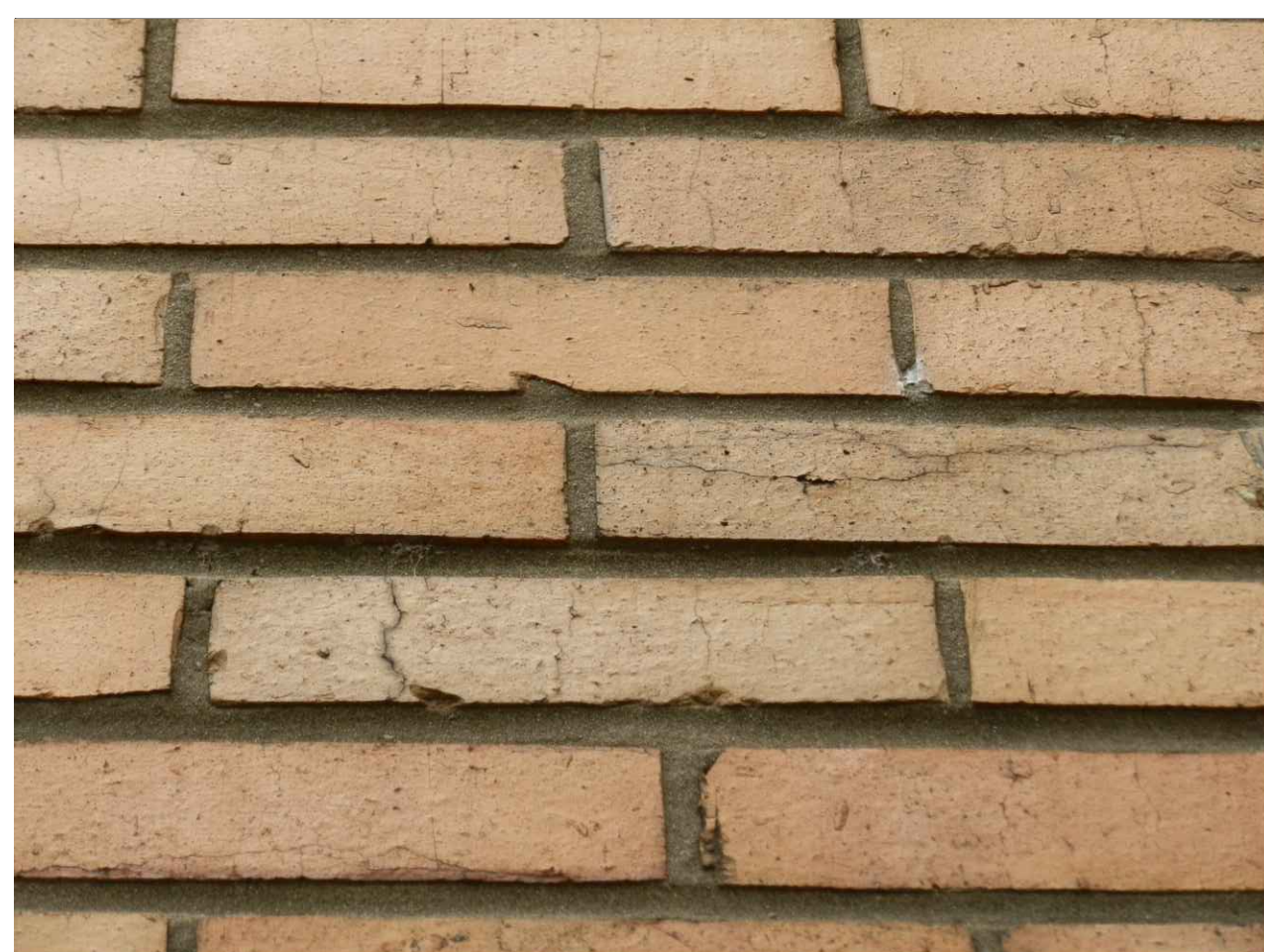
CRACKED AND SPALLING FACE BRICK
