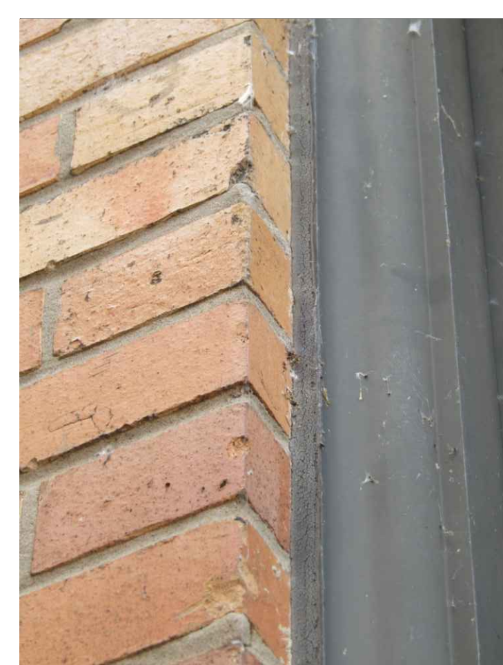
CRACKED AND DETERIORATED WINDOW FRAME SEALANT
