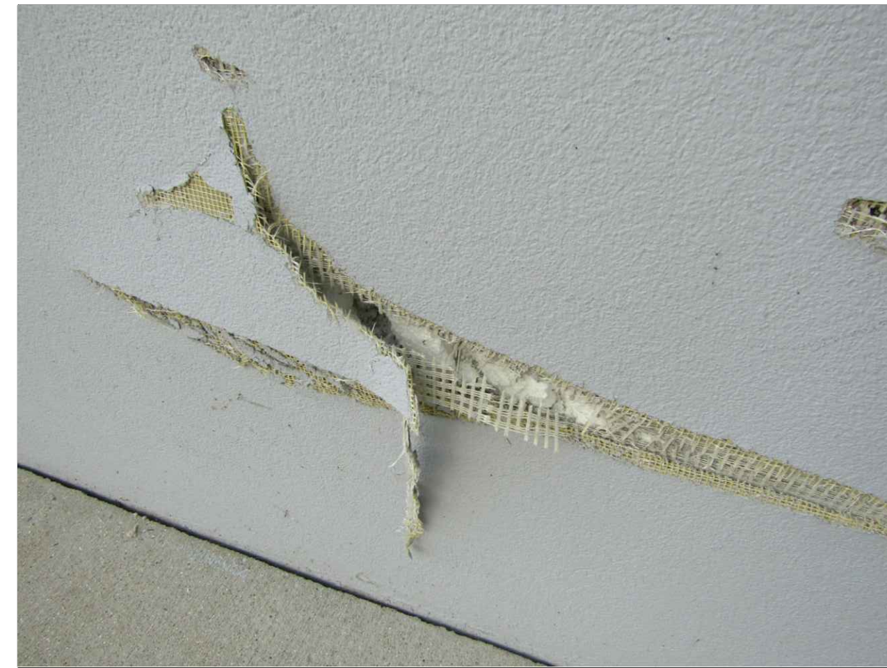
EIFS DAMAGE AND DETERIORATION AT THE WOMEN'S HOSPITAL
