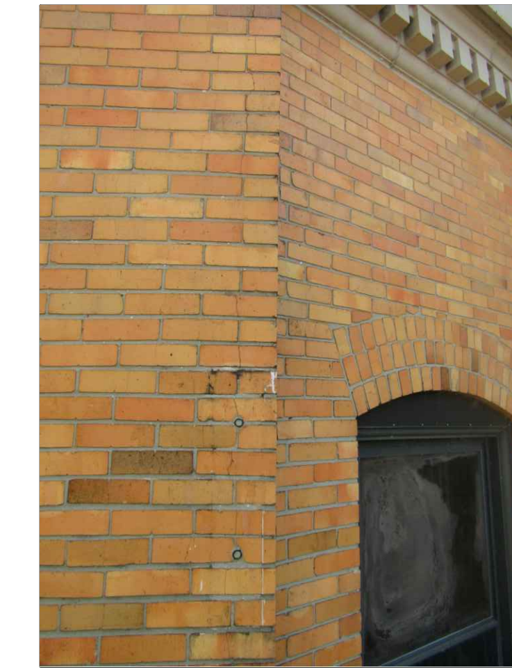
FACE BRICK CRACKING AT CORNER
