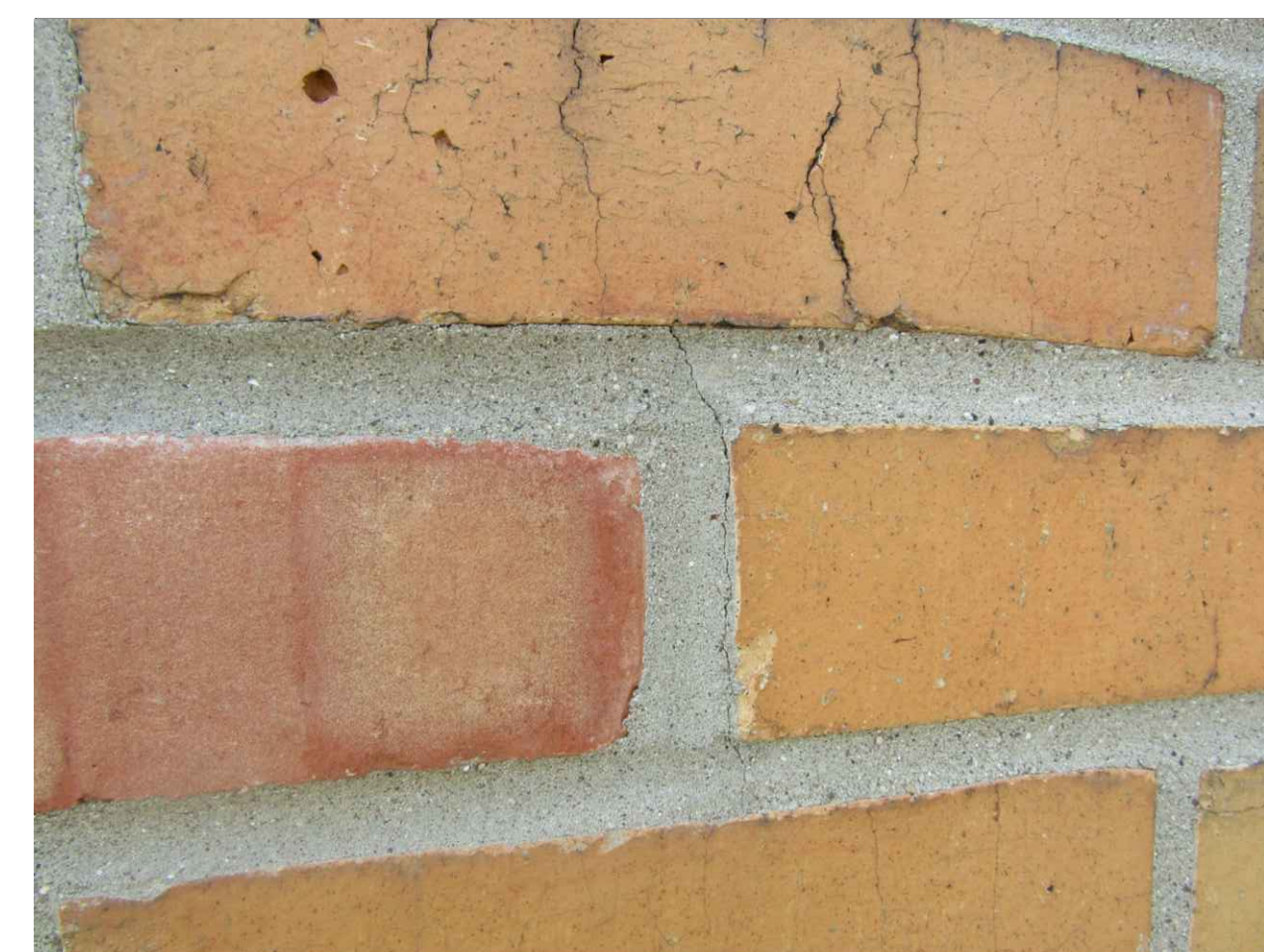
CRACKED AND DETERIORATED MORTAR JOINTS
