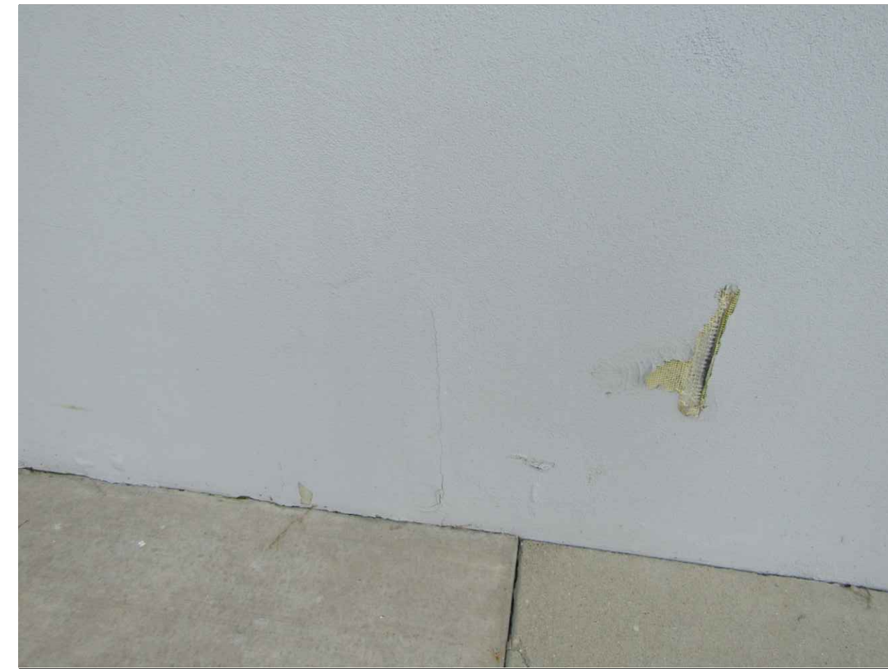
EIFS DAMAGE AND DETERIORATION
