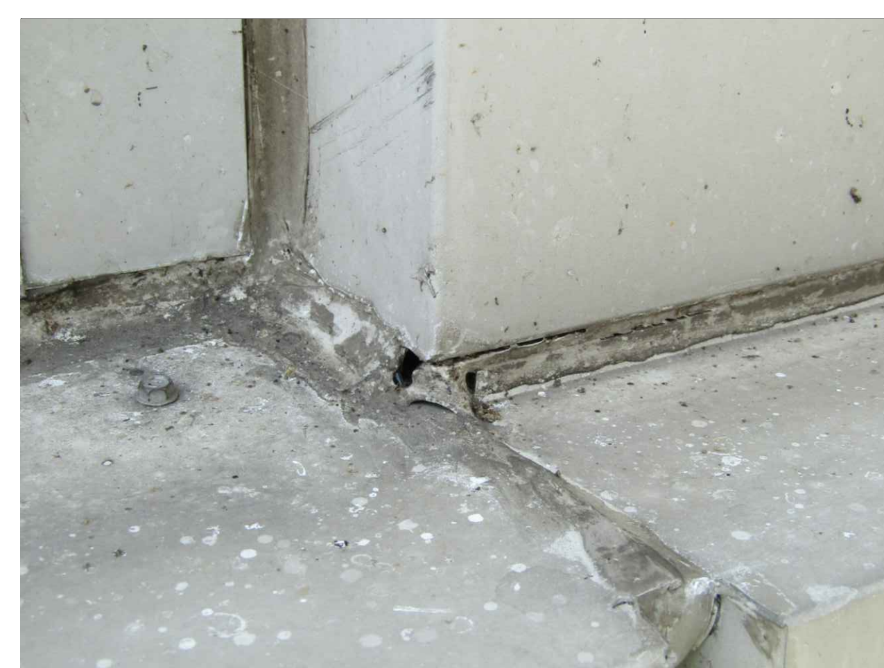
CRACKED AND DEBONDED FRAME SEALANT
