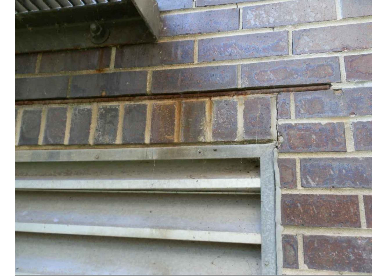
MORTAR DETERIORATION DUE TO CORROSION AT LINTEL
