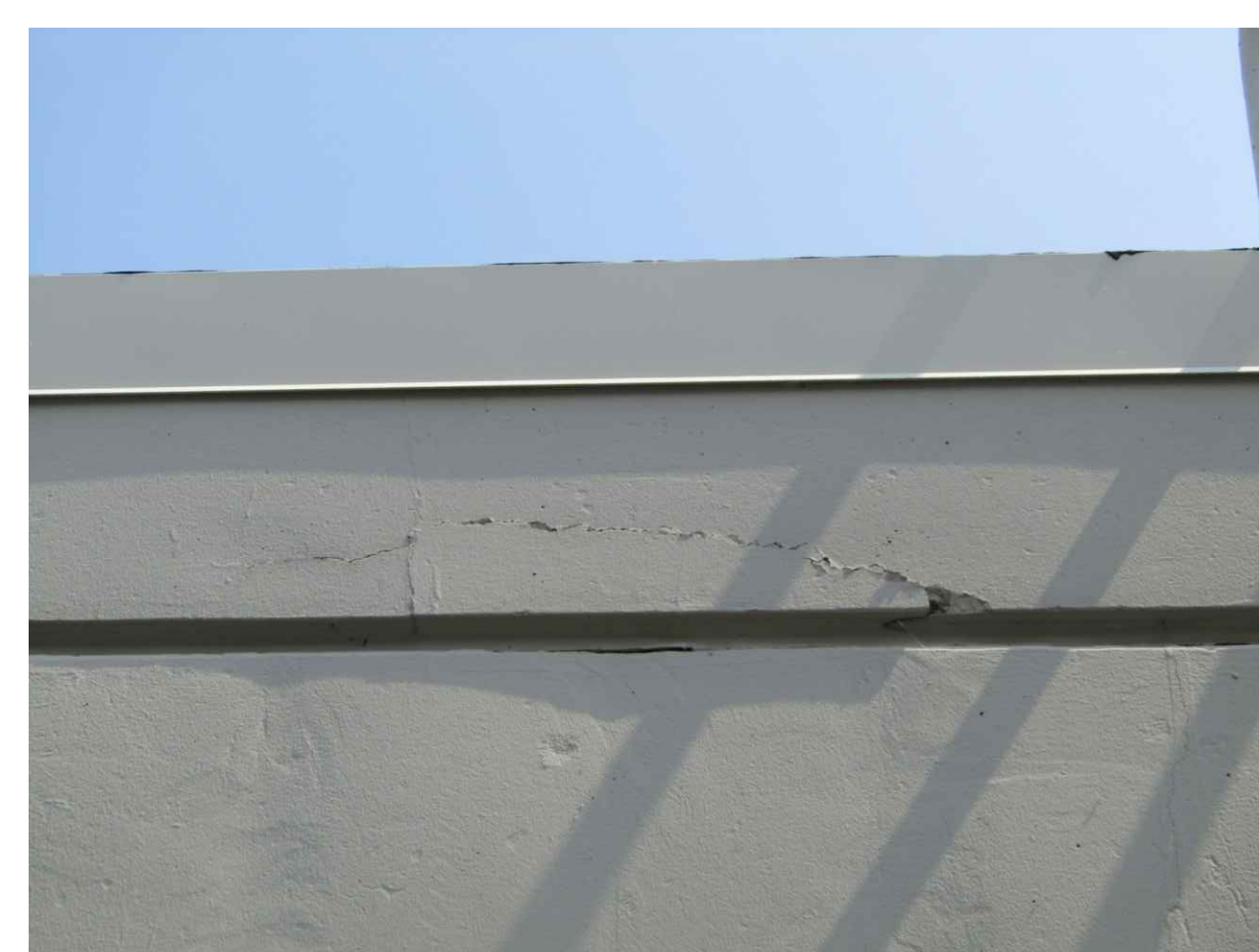
SPALLING AT PRECAST CONCRETE PANEL AT THE WOMEN'S HOSPITAL
