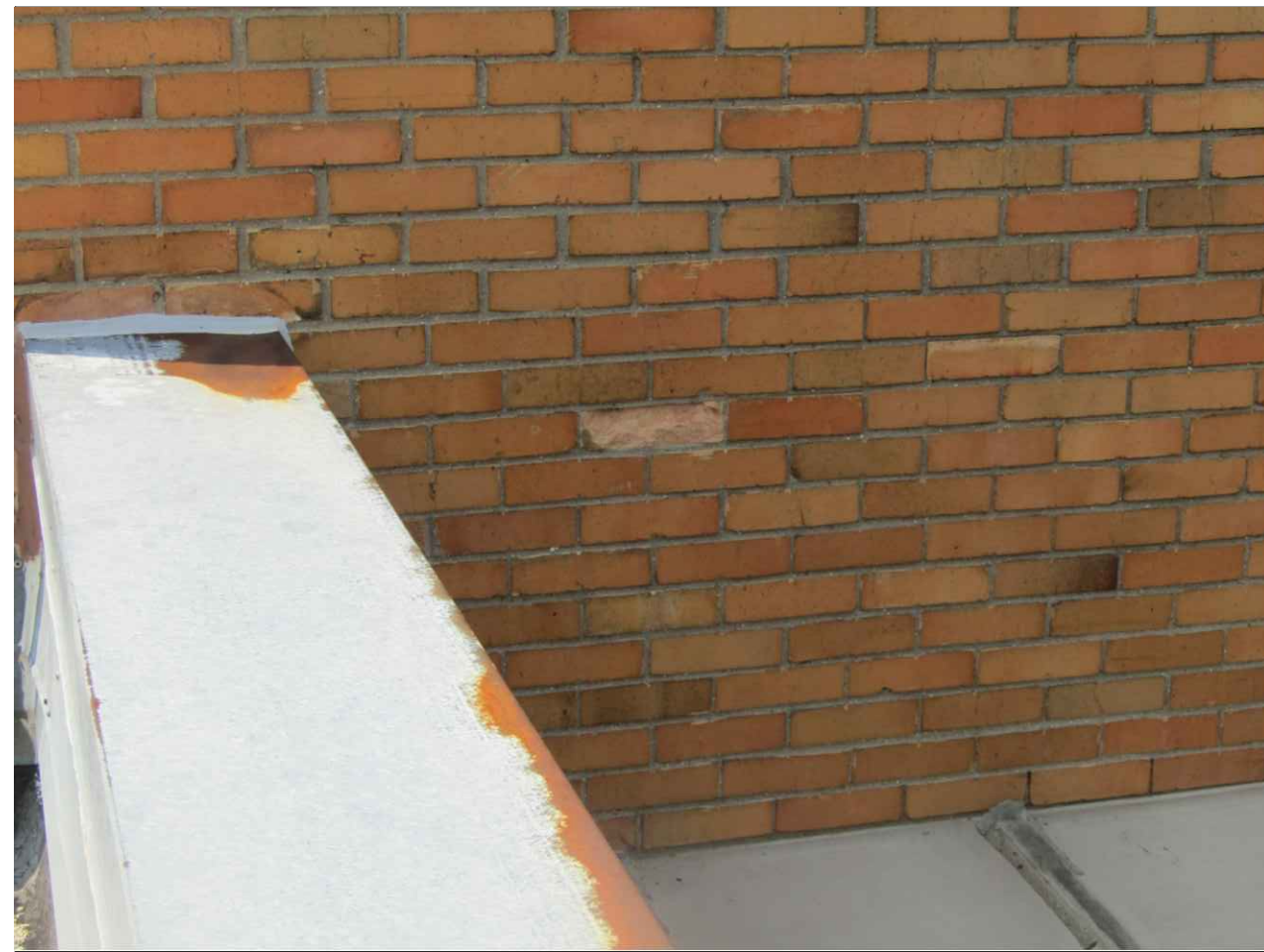
SPALLED FACE BRICK
