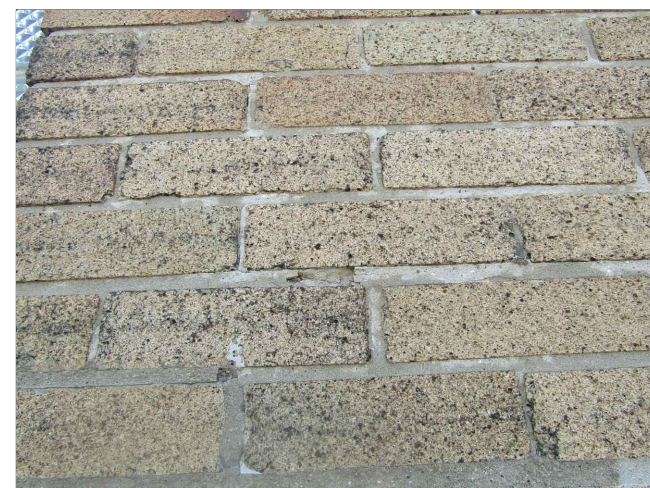
DETERIORATED MORTAR JOINTS
