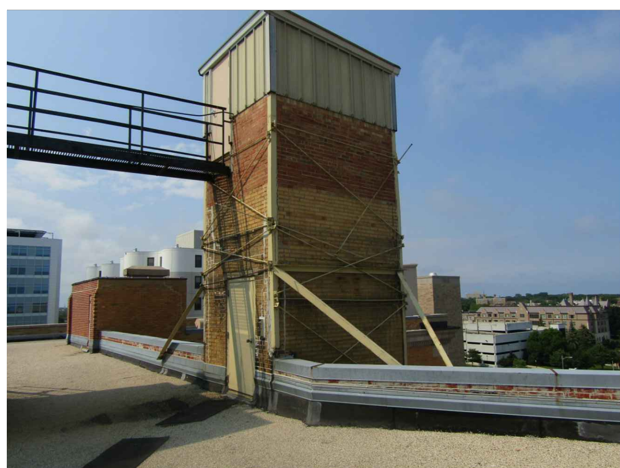
HEAVILY DETERIORATED AND SHORED ELEVATOR SHAFT AT THE HERITAGE CENTER
