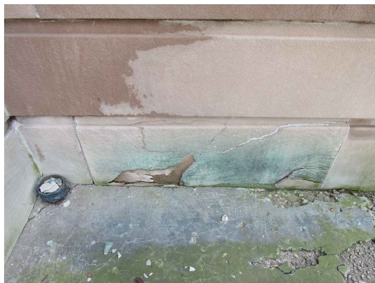
SPALLING AND STAINING AT STONE PANELS AT THE HERITAGE CENTER BUILDING
