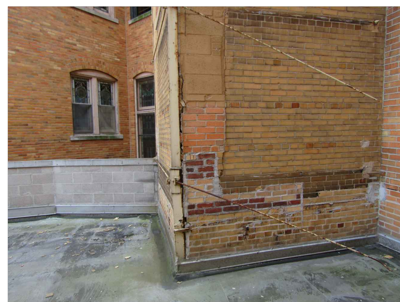
CRACKED AND DETERIORATED FACE BRICK AT ELEVATOR SHAFT
