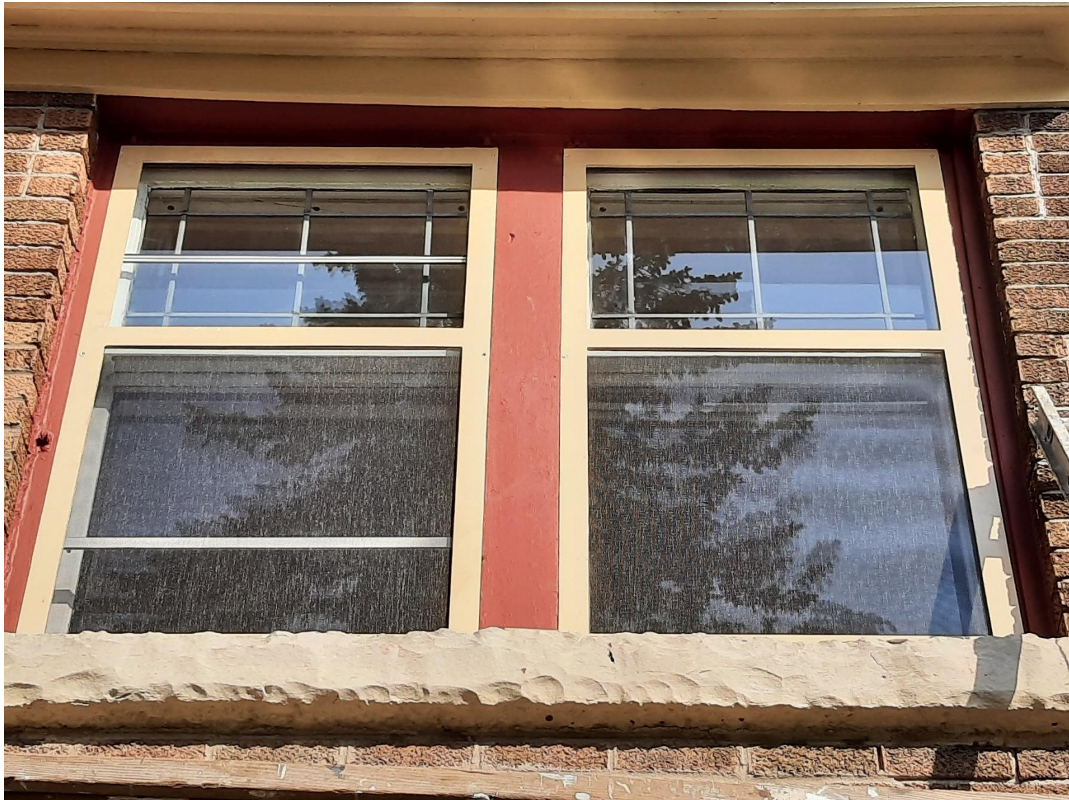
Sample of replica windows and storms. As of 12/20/2022 all second floor front windows match this approved design. Storm window frames still must be painted.
