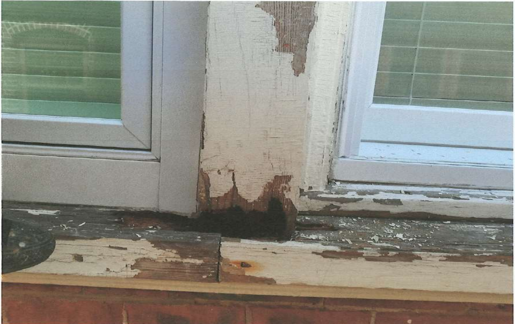
Typical window conditions before work.
