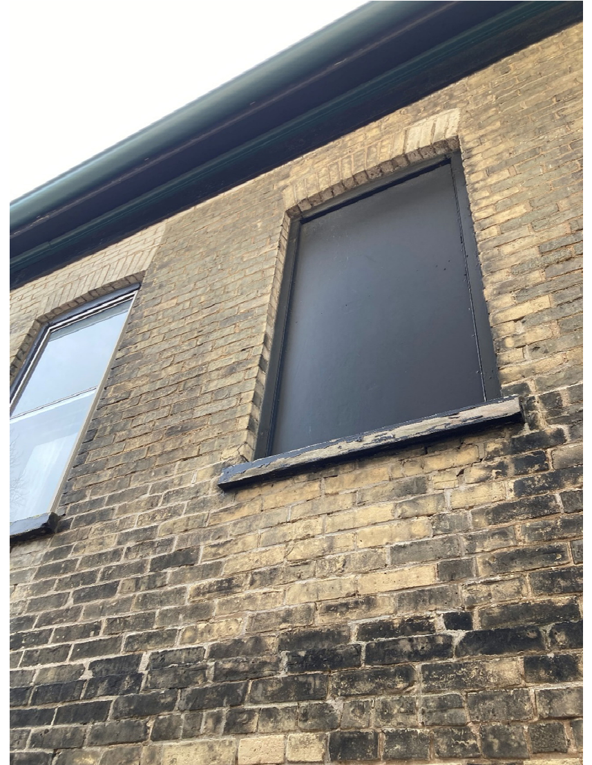
Wooden Sills to be replaced with Stone. Closed Window to be opened. New window to be installed. (North Face)
