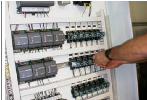
Digital Building Controls
