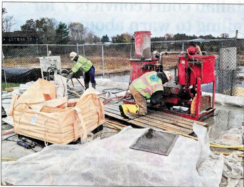
Don Helfenstein, 54 of Burlington, (right), and James Peloquin, 31 of Cambridge, fill in concrete as part of the repairs to the McDill Pond Dam on Monday. B.C. KOWALSKI/JOURNAL STAFF
