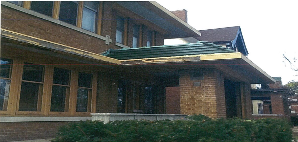
EAST SIDE REPLACE DEFECTIVE BOARDS ON ROOF EAVE
