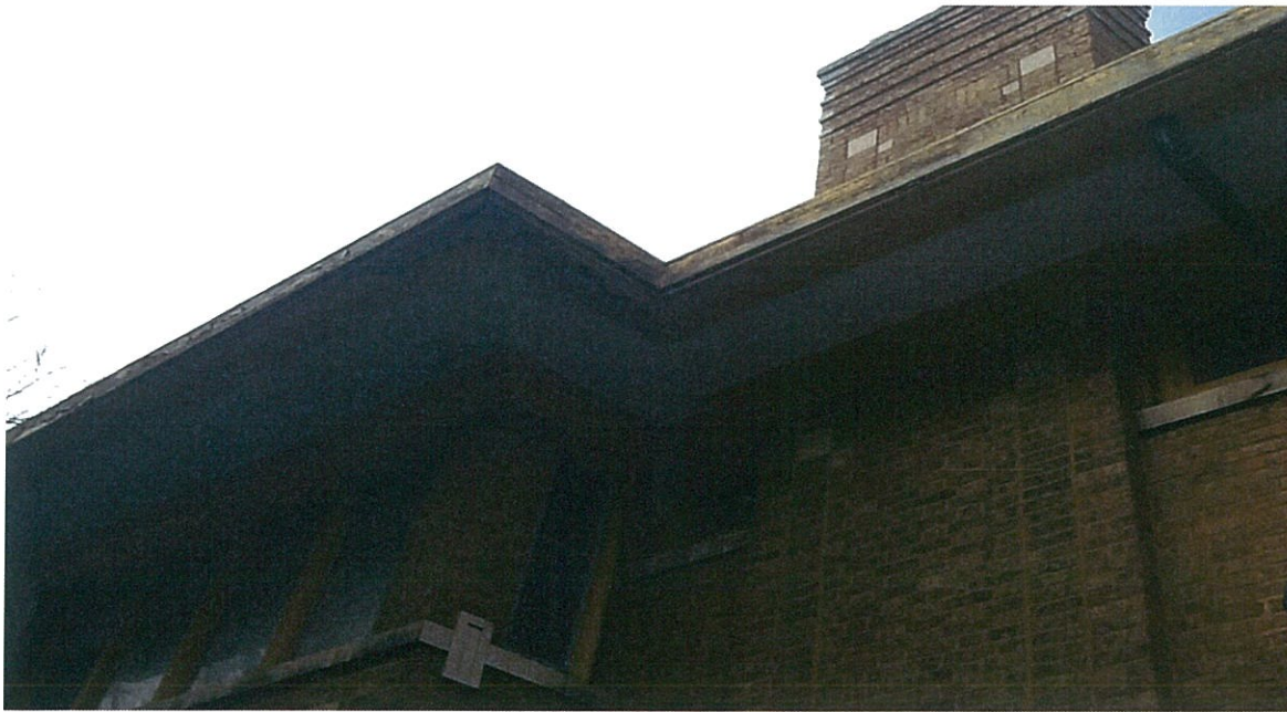
SOUTH SIDE REPLACE DEFECTIVE FACIA BOARDS
