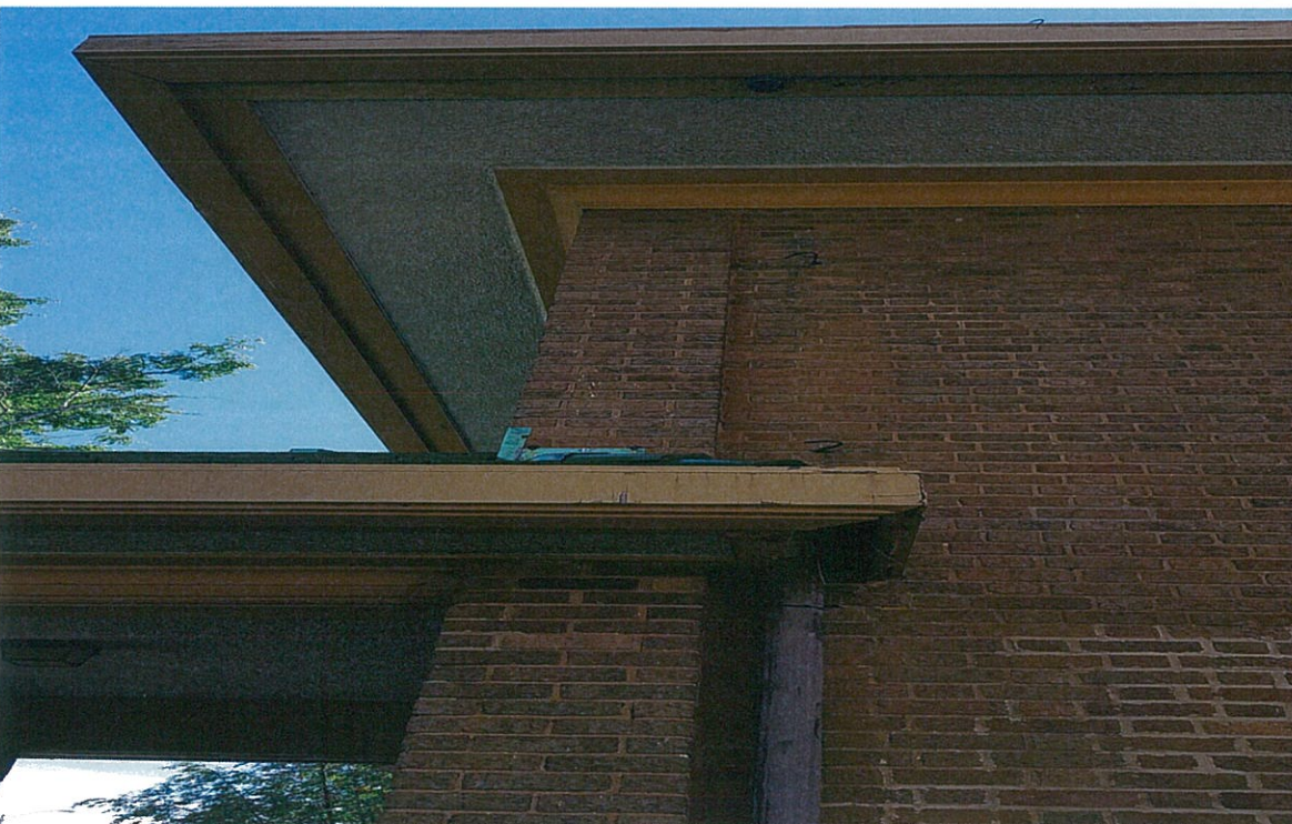
NORTH SIDE REPLACE MISSING DOWNSPOUT
