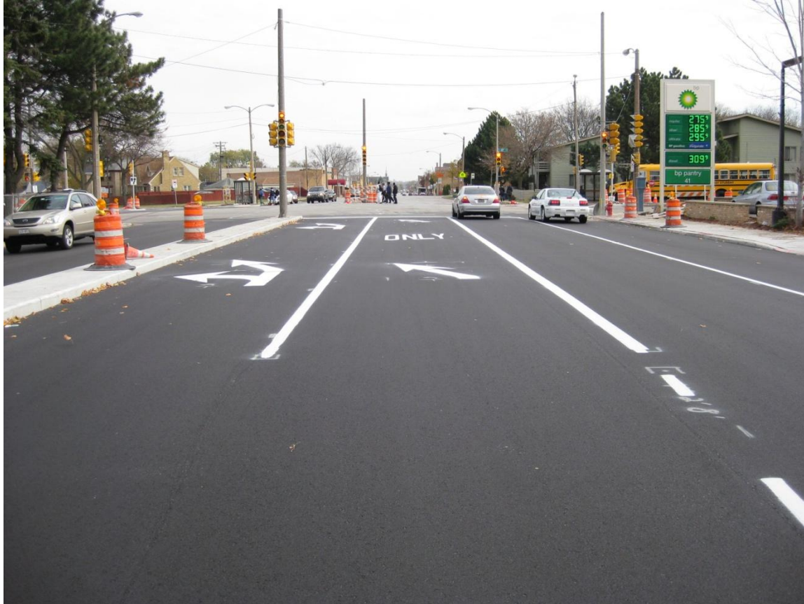
W. Burleigh St. Intersection At N. 60 th St. – Funded by Highway Safety Improvement Program (HSIP)
