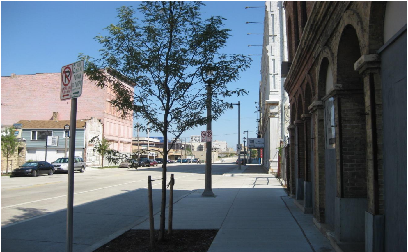
S. 2 nd St. – W. National Ave. to the Milwaukee River: Major Arterial project, Funded by State Transportation Fund (STP)
