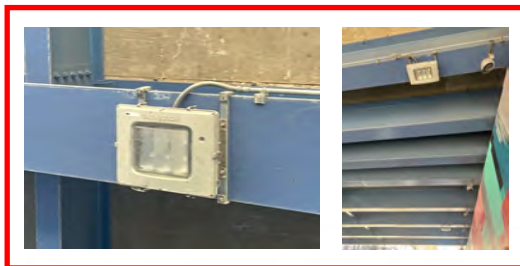
photo example: light fixture at Water Street & Broadway
