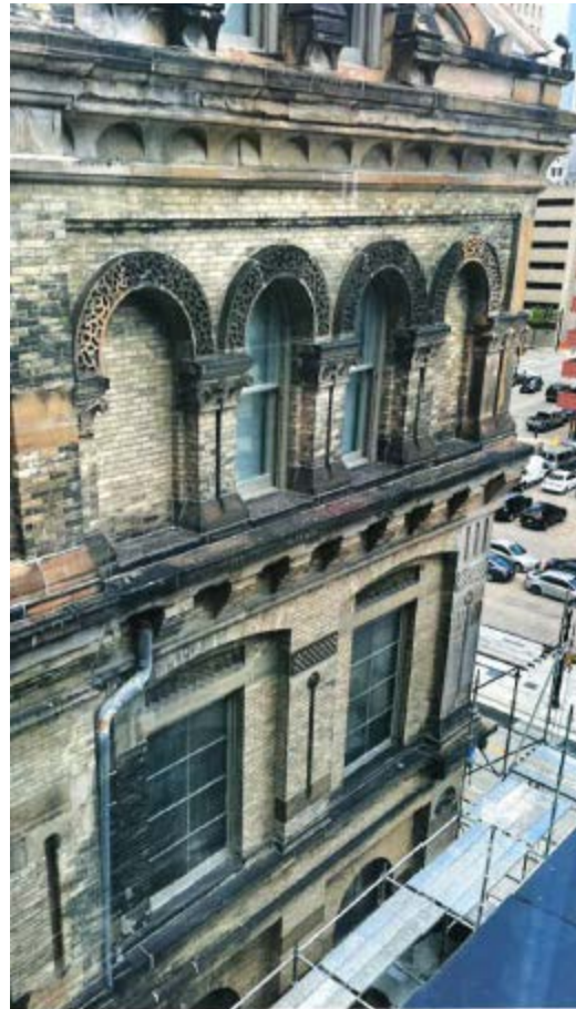
Windows to be painted
