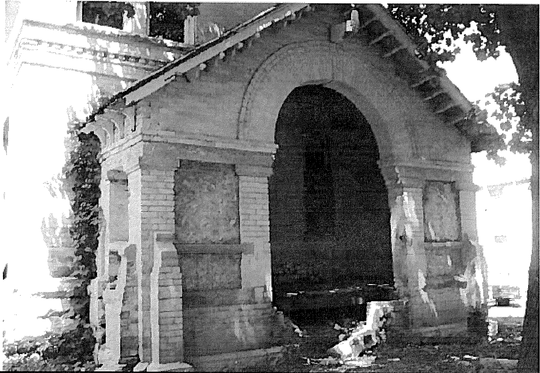
Brick front porch to be carefully dismantled and rebuilt on new foundation. Measured drawings of the porch must be made and approved by HPC staff prior to general construction.
